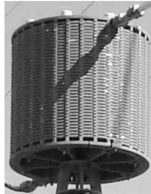
Figure 7 – HV line trap
