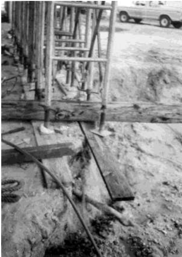
Figure 2.2.3-1—Washout under Sill Support
