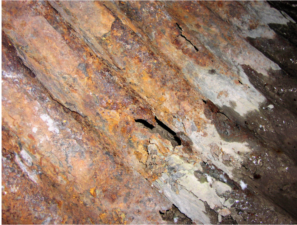
Figure 2.3.1.1-1—Severe Corrosion of Corrugated Steel Culvert
