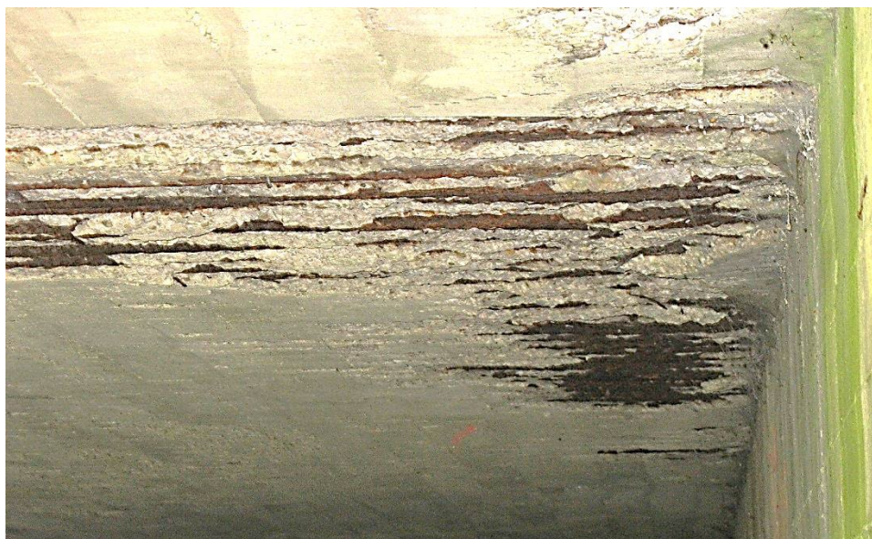
Figure 2.3.1.2.7-1—Corrosion of Reinforcing Steel in Soffit of Concrete Box Culvert
