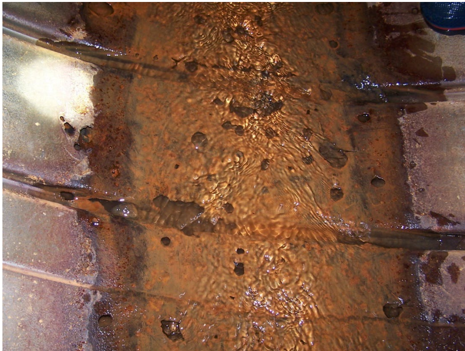
Figure 2.3.1.1-2—Steel Culvert with Invert Perforations
