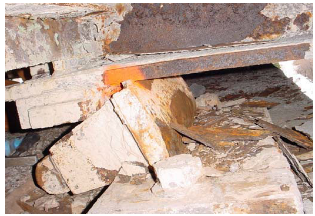
Figure C3.2.3.3-4—Rocker Bearing Failure as a Result of Excessive Leaning Caused by Build-Up of Debris and Corrosion between the Bearing Bottom Surface and Bearing Plate
