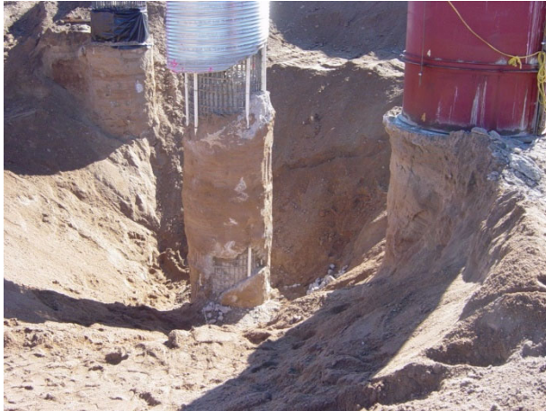
Figure C3.2.3.6-6—Excavated Drill Shaft Showing Cover Defect (Photo Courtesy of NCS GeoResources, LLC)
