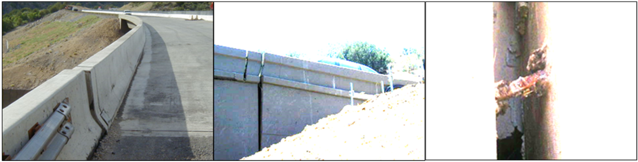
Figure C3.2.3.6-5—Outward Movement of Wing Wall Leading to Reinforcement Pull-Out and Corrosion (Photos Courtesy of NCS GeoResources, LLC)
