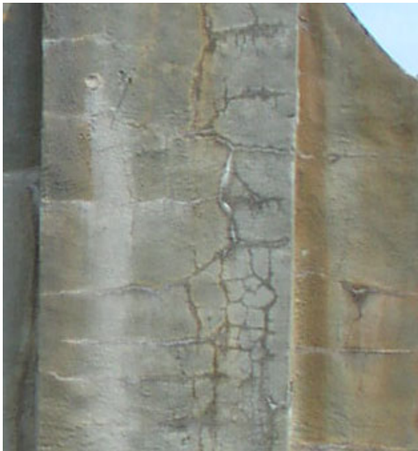
Figure C3.2.3.4-5—Cracked Concrete Abutment Attributed to Reactive Aggregate
