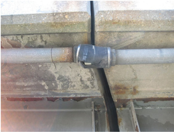
Figure C3.2.3.7-1—Deflection of a Utility Line at a Deck Joint Causing Damage to the Utility Fitting
