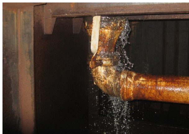
Figure C3.2.3.1-4— Clogged and Leaking Drain (FHWA, 2015)
