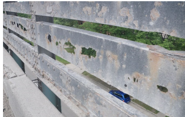
Figure C3.2.3.7-4—Corrosion of Steel Railing Due to Lack of Paint Maintenance Resulting in Section Loss
