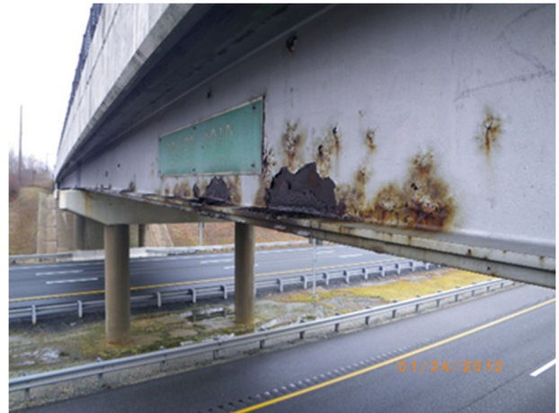
Figure C3.2.3.5-2—Local Corrosion and Paint Failures Within a Splash Zone
