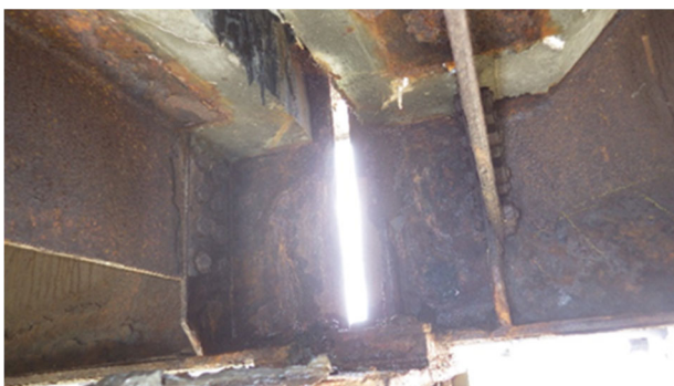
Figure C3.2.3.5-13—Leaking Deck Joint Leading to Loss of Patina and Corrosion of Weathering Steel
