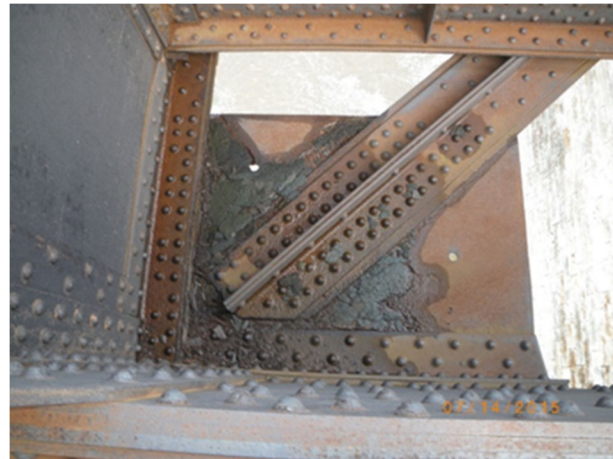
Figure C3.2.3.5-8—Debris on Lateral Gusset Plate Leading to Local Corrosion and Section Loss
