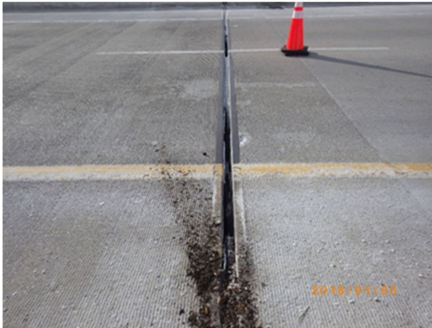
Figure C3.2.3.3-1—Damaged Strip Seal Joint Clogged with Debris
