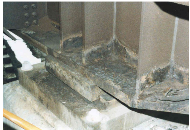
Figure C3.2.3.5-4—Debris and Moisture Traps Formed by Bearing Stiffeners without Drain Holes (FHWA, 2015)
