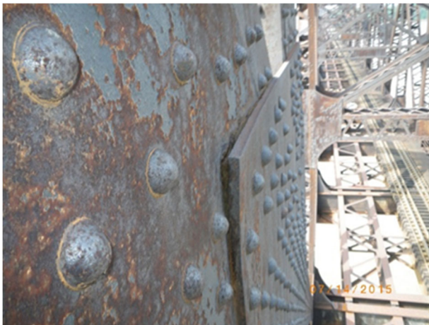
Figure C3.2.3.5-3—Crevice Corrosion Resulting In Distorted Gusset Plate, and Local Corrosion and Paint Failures
