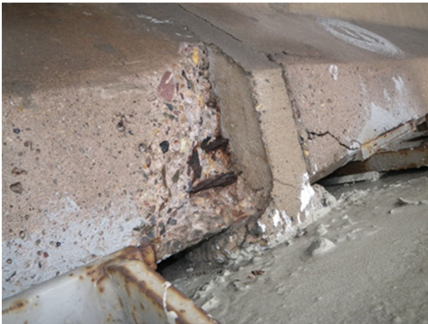
Figure C3.2.3.4-1—End of a Prestressed Concrete Beam with Corroded Strands that Have Caused Cracking and Spalling of Concrete
