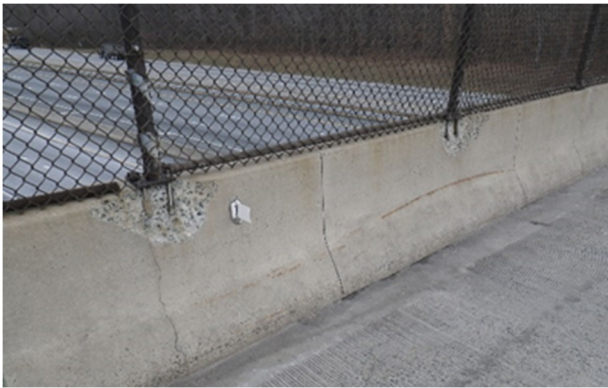
Figure C3.2.3.7-3—Parapet with Spalled Concrete at the Anchor Bolts Attaching a Pedestrian Fence
