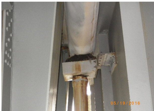
Figure C3.2.3.1-3—Drain Pipe beneath a Joint Clogged with Debris
