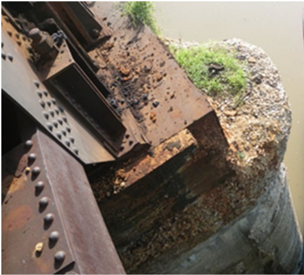
Figure C3.2.3.4-7—Concrete Surface Scaling Attributed to Freeze–Thaw
