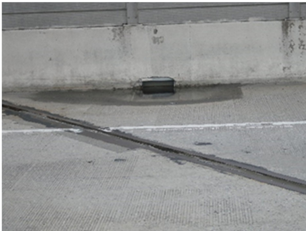
Figure C3.2.3.2-3—Ponding on a Deck Surface Near a Scupper
