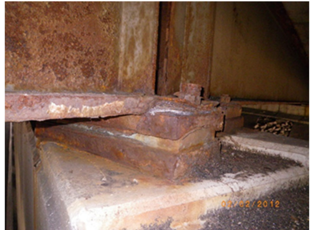
Figure C3.2.3.3-2—Corroded Steel Bearing Attributed to Leaking Joint
