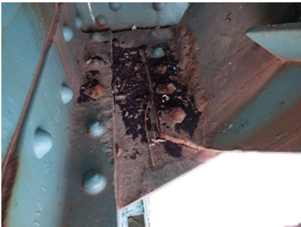
Figure C3.2.3.5-9—Moisture and Debris on Lateral Gusset Resulting in Corrosion and Section Loss
