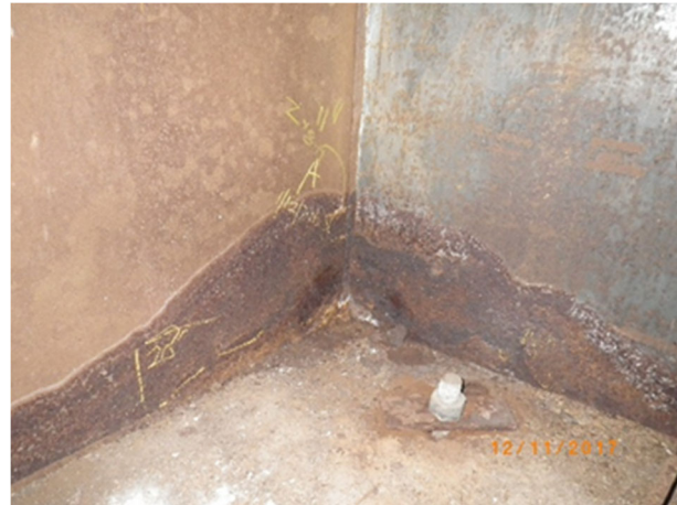
Figure C3.2.3.5-6—Trapped Moisture within a Box Girder Resulting in Local Corrosion
