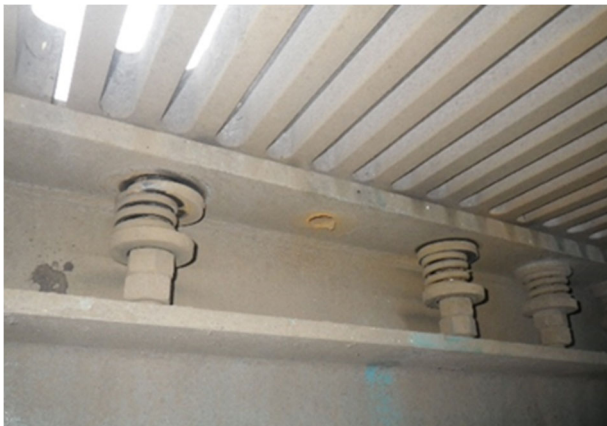
Figure C3.2.3.3-3—Tooth Plate with Missing Bolt. Loss of Bolts Can Result in a Loose Plate that May Cause Damage to Joint and Other Members
