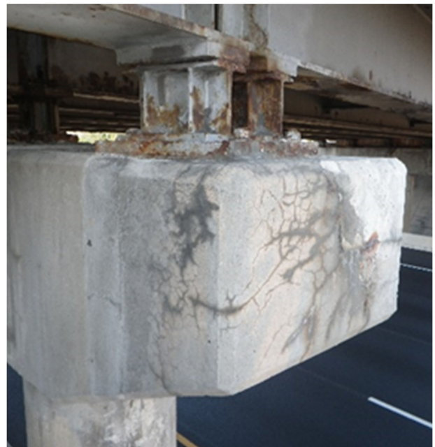
Figure C3.2.3.4-6—Crazeing of Concrete Pier Cap under Roadway Joint Attributed to Reactive Aggregate
