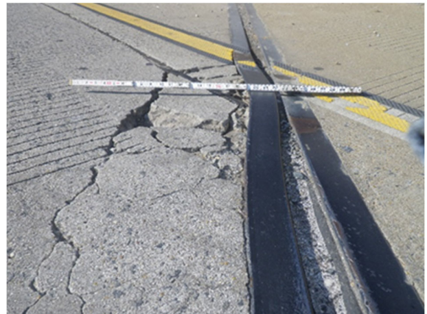
Figure C3.2.3.2-4—Cracked and Spalled Concrete at a Damaged Deck Joint
