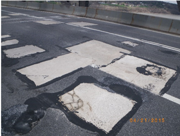
Figure C3.2.3.2-1—Deck Repairs Required by Delamination and Potholes Attributed to Corrosion of Reinforcement
