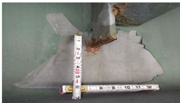
Figure C3.2.3.5-14—Fatigue Crack at the Bottom of a Connection Plate
