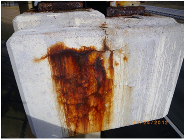
Figure C3.2.3.4-3—Cracked and Delaminated Concrete with Corroded Reinforcement on End of Pier Cap under Roadway Joint
