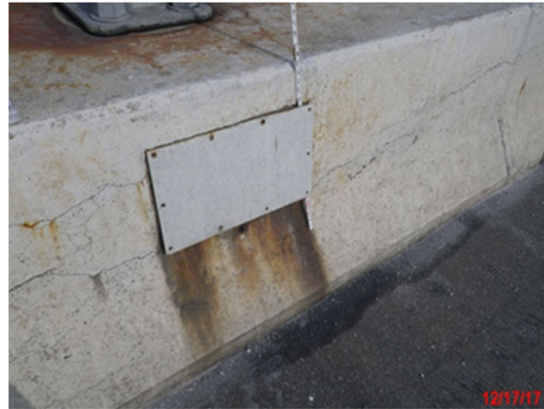
Figure C3.2.3.7-2—Local Cracking and Corrosion in the Area of an Electrical Box within a Parapet Causing Staining of the Concrete
