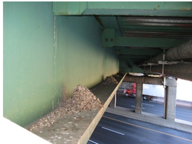
Figure C3.2.3.5-10—Bird Droppings which Entrap Moisture, Often Resulting in Local Corrosion and Section Loss
