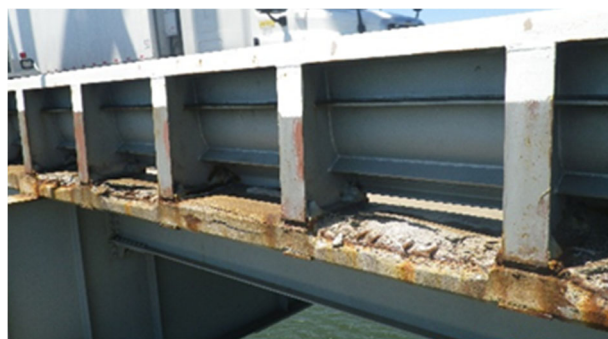
Figure C3.2.3.1-2—Damage to Concrete at Free Drop Deck Drains
