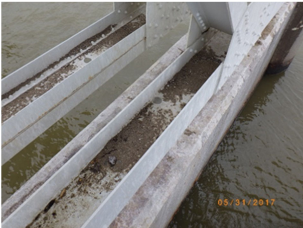
Figure C3.2.3.5-7—Debris Collected Along Horizontal Web of I-Shaped Truss Members, One Welded and One Riveted Built-Up Member. Note No Drain Holes Evident in Picture.
