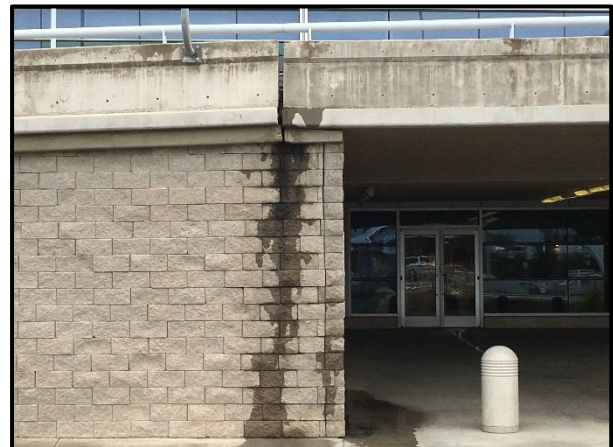
Figure C3.2.3.6-4—Joint Leakage Due to Differential Settlement (Photo Courtesy of NCS GeoResources, LLC)
