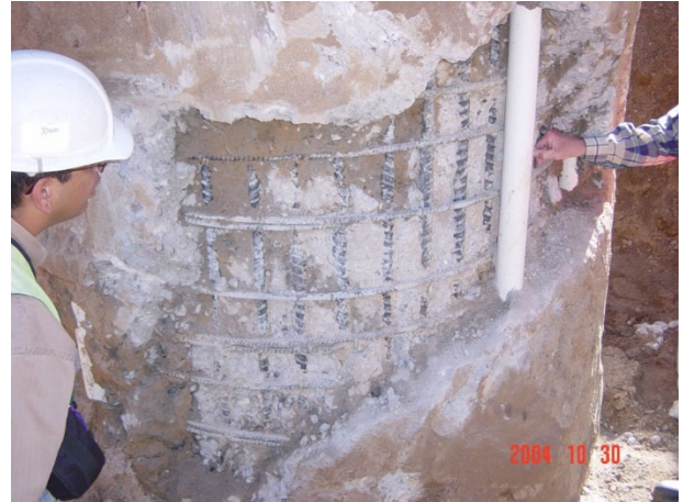
Figure C3.2.3.6-7—Close-Up of Cover Defect (Photo Courtesy of NCS GeoResources, LLC)
