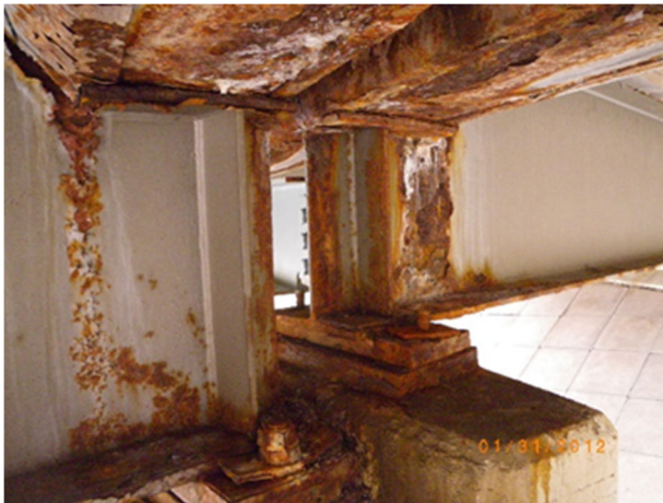
Figure C3.2.3.5-1—Corroded Beam Ends and Bearings Under Leaking Deck Joint and Splash from Drain Pipe
