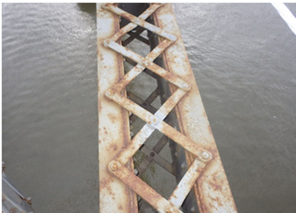
Figure C3.2.3.5-11—Localized Paint Failures and Corrosion on Built-Up Truss Member
