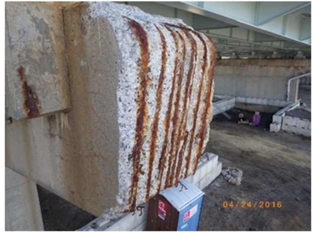
Figure C3.2.3.4-4—Spalled Concrete and Corroded Reinforcement at End of Pier Cap. Condition Shown in Figure 3.2.3.4-3 May Reach this Stage If Not Addressed
