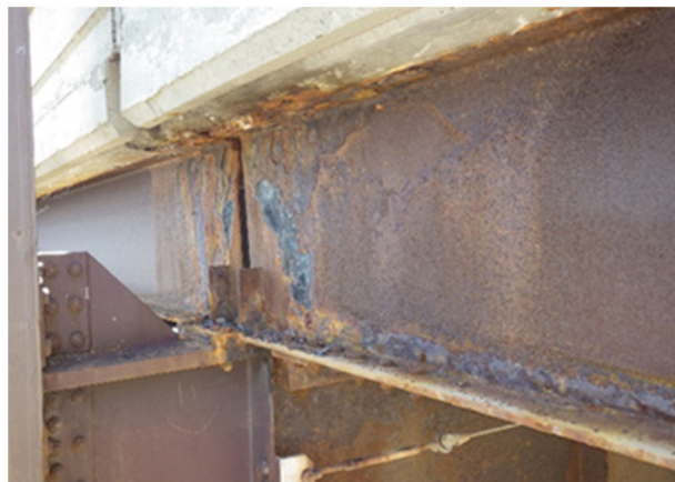
Figure C3.2.3.5-12—Loss of Patina on Weathering Steel Girders Leading to Corrosion
