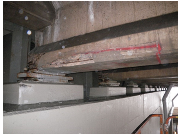
Figure C3.2.3.4-2—Ends of Prestressed Concrete Beams Showing Delaminated Concrete and Exposed, Corroded Strand Attributed to Exposure to Roadway Drainage
