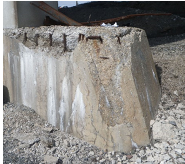
Figure C3.2.3.4-8—Deteriorated Concrete Footing with Exposed Reinforcement. Possible Sources Include Reactive Aggregate and Freeze–Thaw.
