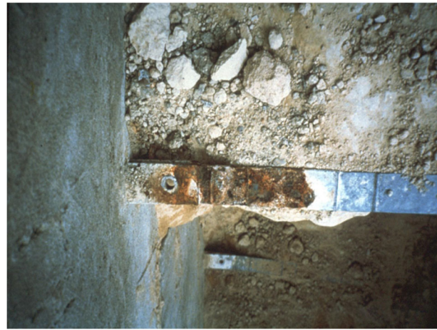
Figure C3.2.3.6-2—Corroded Steel Soil Reinforcing Strip Exposed behind MSE Wall Attributed to Runoff Containing Deicing Salt. A Membrane is Now Required at Top of Reinforced Fill to Address this Situation (Photo Courtesy of FHWA)
