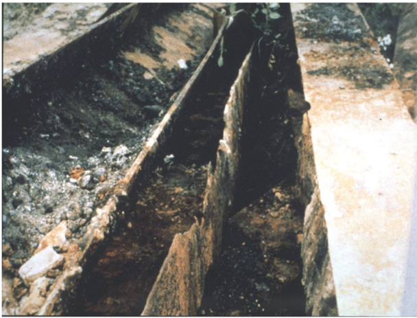
Figure C3.2.3.6-1—Corrosion of Steel H-Pile Taken out of Service (Photo Courtesy of FHWA)
