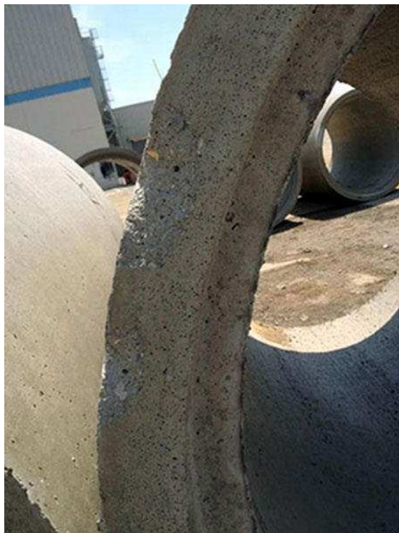
Figure 9 —Acceptable Chip on Bell End ( Photo Courtesy of ACPA )
