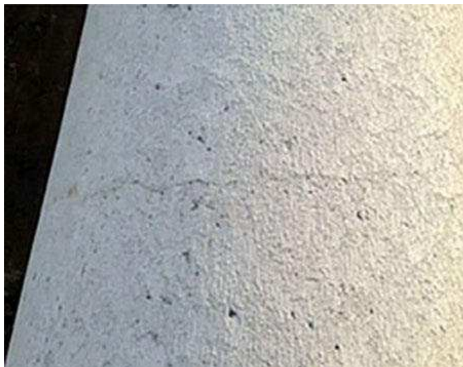
Figure 4 —Acceptable Surface/Curing Crack ( Photo Courtesy of ACPA )
