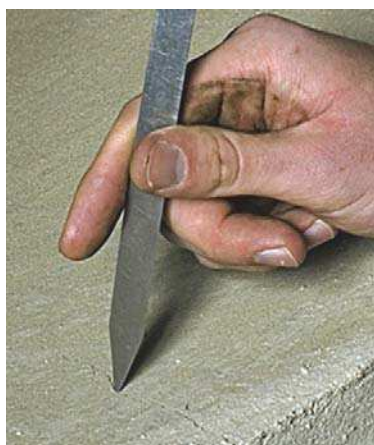
Figure 2 —0.01-in. Crack Measurement (Photo Courtesy of ACPA)
