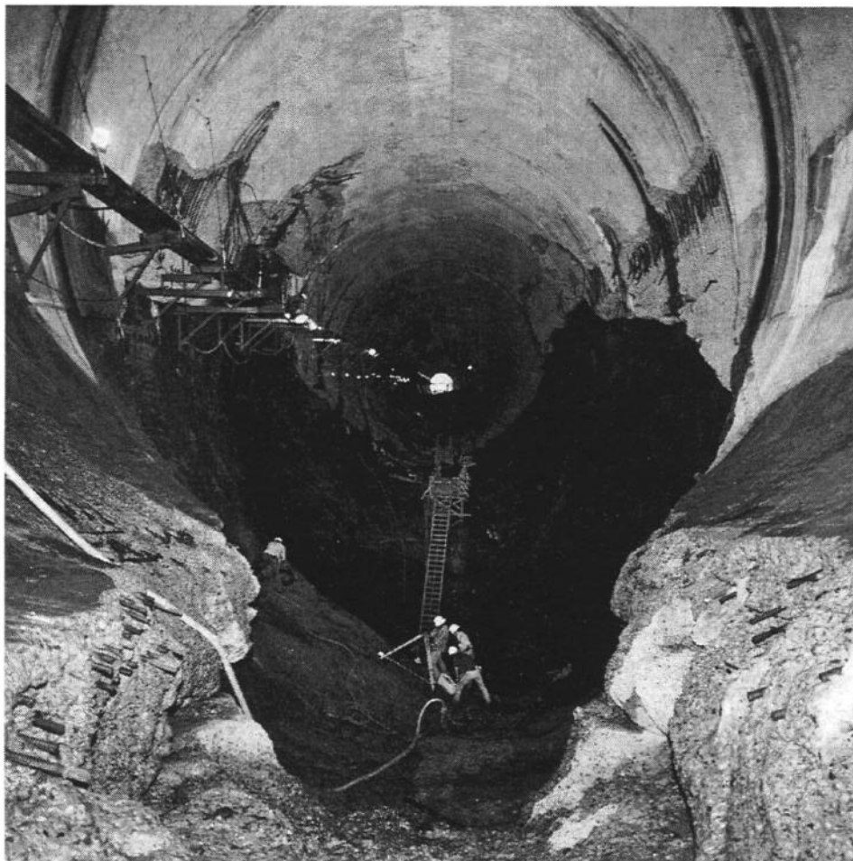
Fig. 2.3-Glen Canyon Dam. Erosion of spillway tunnel invert and sandstone foundation rock downstream of the elbow
