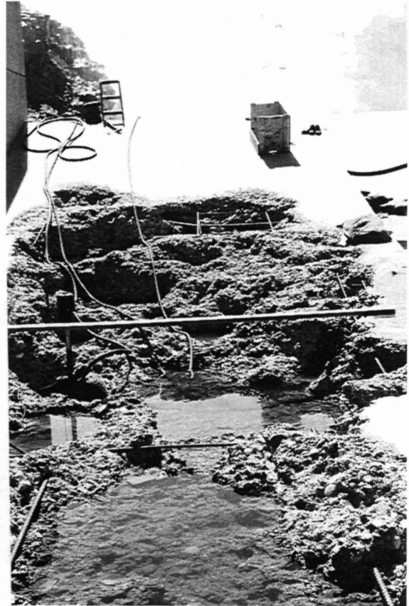
Fig. 2.6-Lucky Peak Dam. Cavitation erosion of flip lip surface
