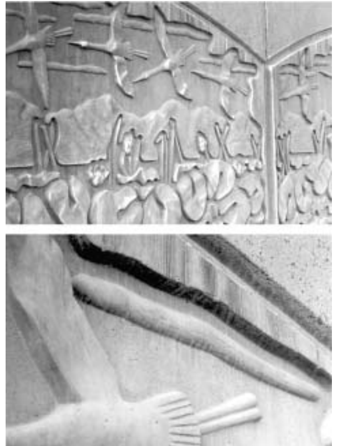
Fig. 1.1(c)—Close-ups of surfaces resulting from good consolidation.
