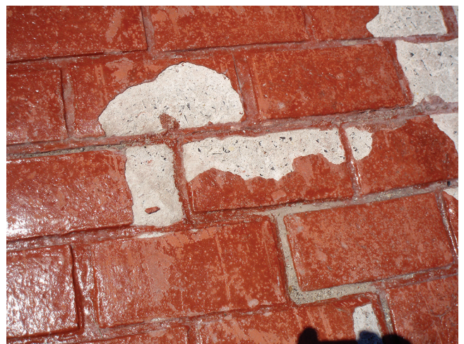
Fig. 4.3c—Delamination of color shake-on hardener illustrating depth of coloration (courtesy of Patterned Concrete of Pennsylvania Inc.).
