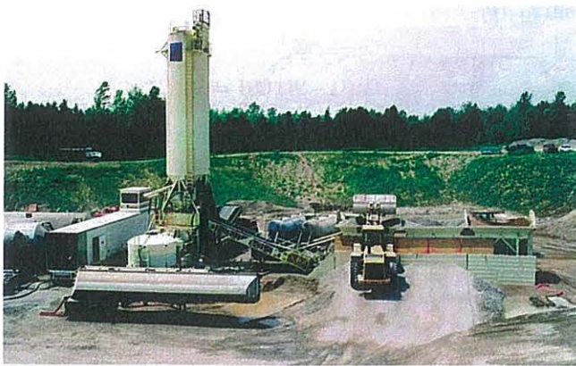
Fig. 4.4—Concrete mixing plant and aggregate storage. Bins contain different size aggregates.
