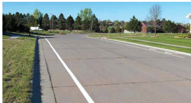
Fig. 4.5—Example of RCC pavement used for a local street (Harrington et al. 2010).
