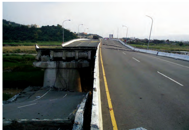
Fig. 1.2.1c—Unseating of bridge deck, JiJi earthquake (Kochi University of Technology 2008).
