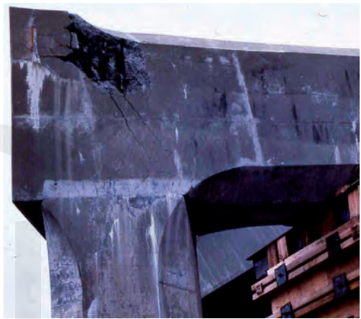
Fig. 1.2.3—Bridge joint damage, 1989 Loma Prieta earthquake (Priestley et al. 1996).
