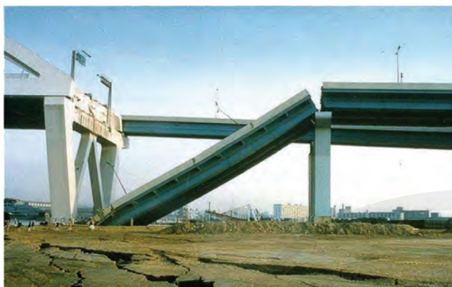
Fig. 1.2.1b—Unseating of Nishinomiya-Ko Bridge approach span during 1995 Kobe earthquake. (University of Washington 2008).
