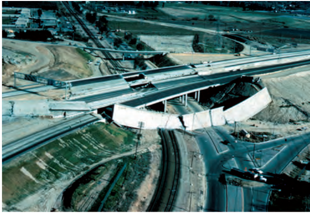
Fig. 1.2a—1971 San Fernando Earthquake.
