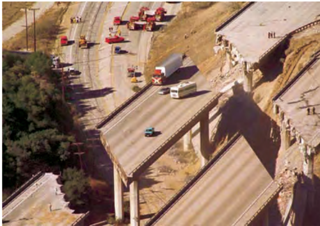
Fig. 1.2.1e—Unseating of skewed bridge, freeway collapse, Northridge earthquake (Heney et al. 1999).
