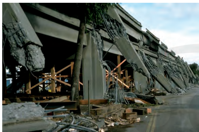
Fig. 1.2.4b—I-880 Cypress double deck viaduct after failure, 1989 Loma Prieta earthquake.
