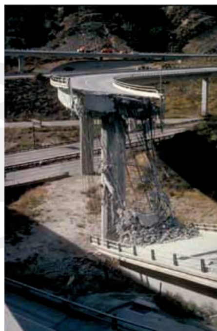
Fig. 1.2.1d—Unseating of curved bridge, I-5 Antelope Valley Freeway collapse, Northridge earthquake (USGS 1996).
