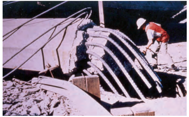
Fig. 1.2.2c—Anchorage failure of column bars, 1971 San Fernando earthquake (Priestley et al. 1996).
