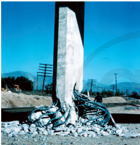
Fig. 1.2.2a—Inadequate confinement, 1971 San Fernando earthquake (USGS 2008b).
