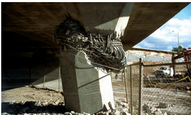
Fig. 1.2.2b—Shear failure, 1994 Northridge earthquake (FEMA 2009a).
