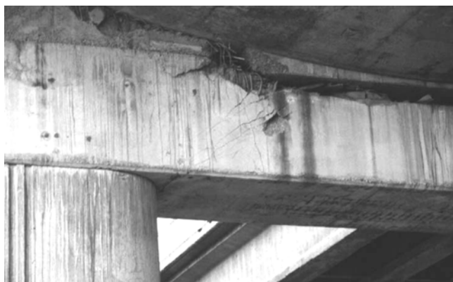
Fig. 2.7—Cap beam damage in 1999 Chi-Chi earthquake. (Courtesy of University of Washington.)
