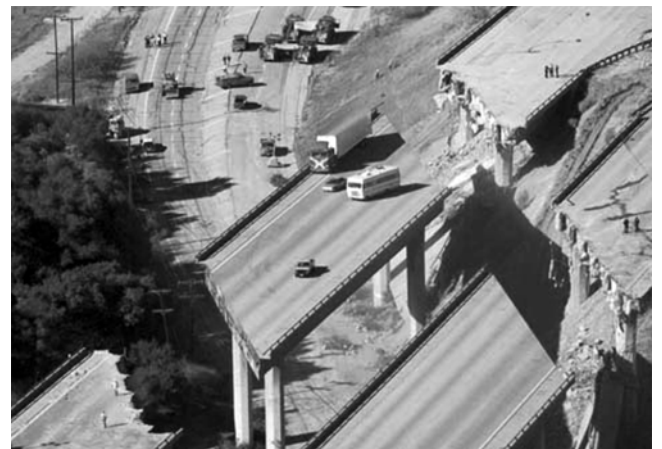
Fig. 2.2—Damage to superstructure due to rotation of skewed spans (courtesy of San Francisco Chronicle).
