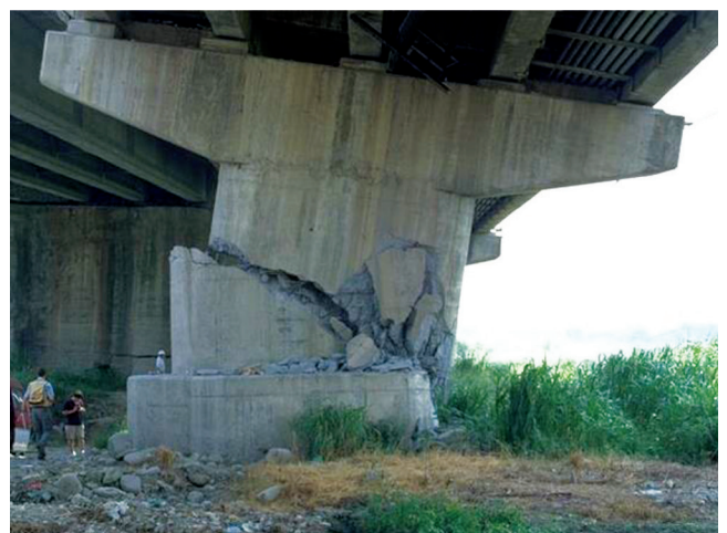
Fig. 4.2.4f—Column shear failure, Wu-Hsi Bridge, 1999 Chi Earthquake. (Courtesy of NISEE, University of California, Berkeley, CA [Moehle 1999b].)
