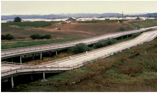
Fig. 4.2.4g—Overview of collapse of Highway 101 at Struve Slough, 1989 Loma Prieta Earthquake. (Courtesy of NISEE, University of California, Berkeley, CA [Boulanger 1989a].)
