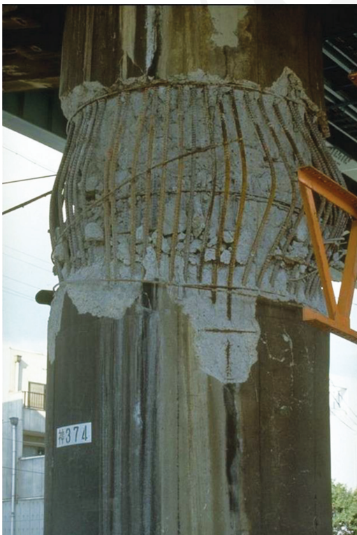
Fig. 4.2.4d—Failure of transverse reinforcement and damage to column core at upper portion of Pier 374 of the Hanshin Expressway, 1995 Kobe Earthquake. (Courtesy of NISEE, University of California, Berkeley, CA [Thewalt 1995f].)
