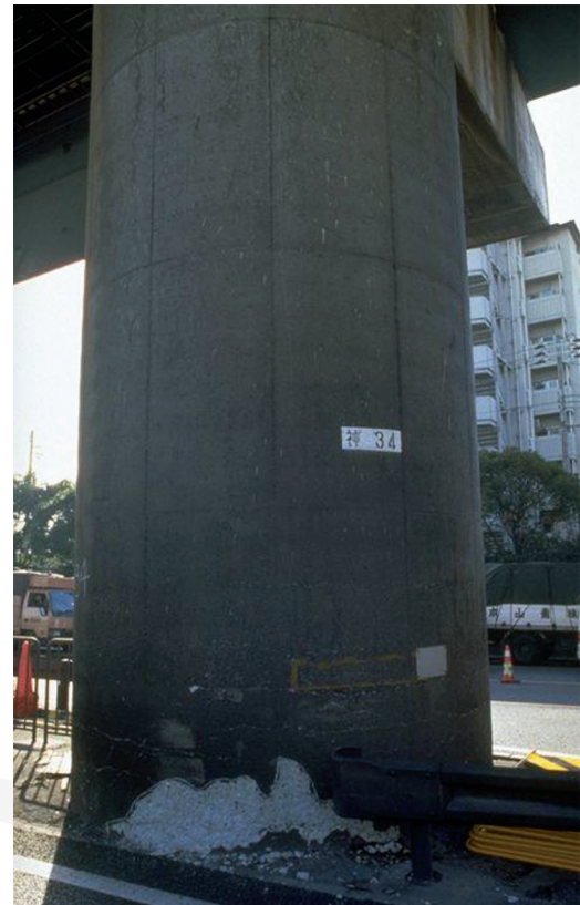
Fig. 4.2.2b—Spalled concrete on the northwest face of Pier 34, Hanshin Expressway, 1995 Kobe Earthquake. (Courtesy of NISEE, University of California, Berkeley, CA [Thewalt 1995c].)
