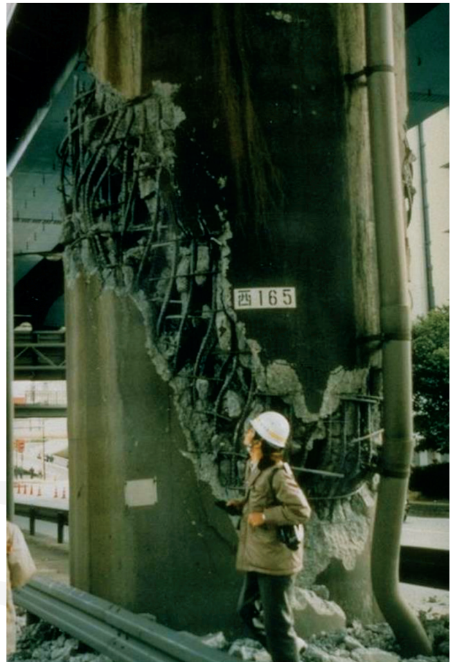
Fig. 4.2.4e—Shear failure of Pier 165, Hanshin Expressway, 1995 Kobe Earthquake. (Courtesy of NISEE, University of California, Berkeley, CA [Thewalt 1995g].)
