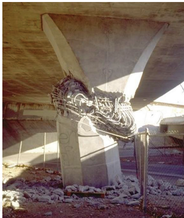
Fig. 4.2.4a—Shear failure at base of column flare, Mission-Gothic Bridge, 1994 Northridge Earthquake. (Courtesy of NISEE, University of California, Berkeley, CA [Aschheim 1994].)
