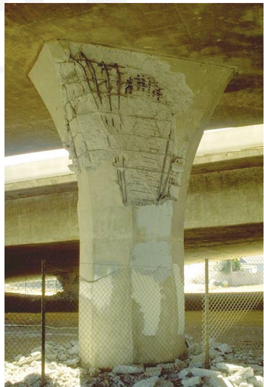
Fig. 4.2.2c—Mission-Gothic Bridge cover spalling, State Route 118, 1994 Northridge Earthquake. (Courtesy of NISEE, University of California, Berkeley, CA [Draher 1994].)
