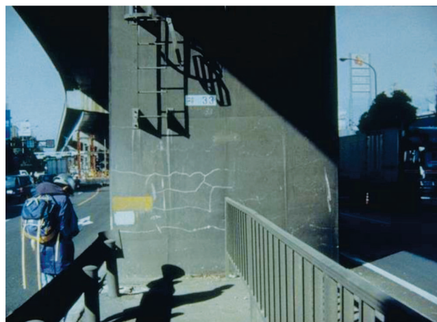
Fig. 4.2.1—East face of Pier 33, Hanshin Expressway, 1995 Kobe Earthquake. (Courtesy of NISEE, University of California, Berkeley, CA [Thewalt 1995a].)
