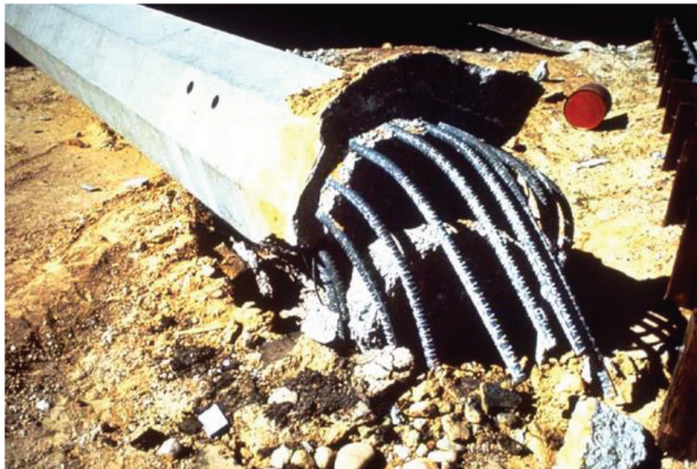
Fig. 4.2.4l—Anchorage failure, Interstate 5/210 interchange, 1971 San Fernando Earthquake. (Courtesy of NOAA/NGDC, U.S. Geological Survey [Leyendecker 1971b].)
