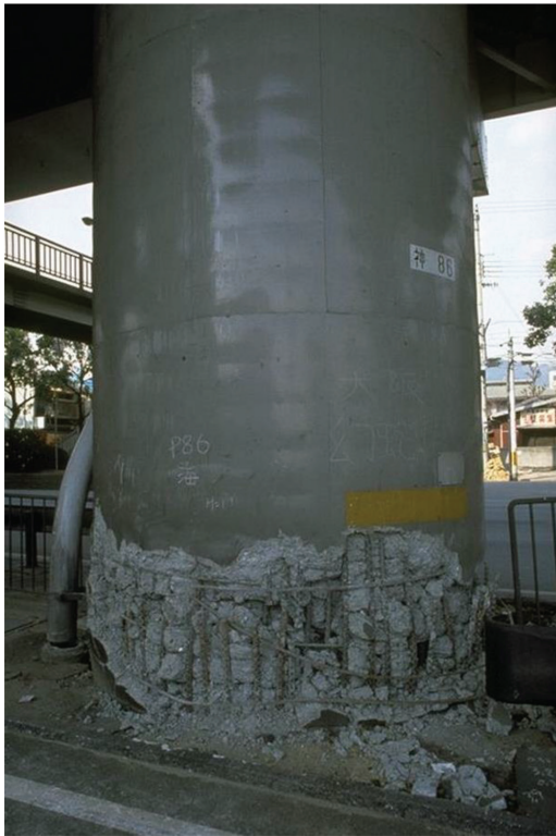
Fig. 4.2.4c—Failure of transverse reinforcement and damage to column core at base of Pier 86 of the Hanshin Expressway, 1995 Kobe Earthquake. (Courtesy of NISEE, University of California, Berkeley, CA [Thewalt 1995e].)
