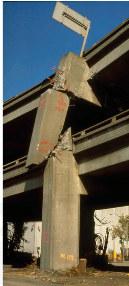
Fig. 4.2.4i—Column and joint failure of double-deck viaduct, I-880, 1989 Loma Prieta Earthquake. (Courtesy of NISEE, University of California, Berkeley, CA [Dickenson 1989].)
