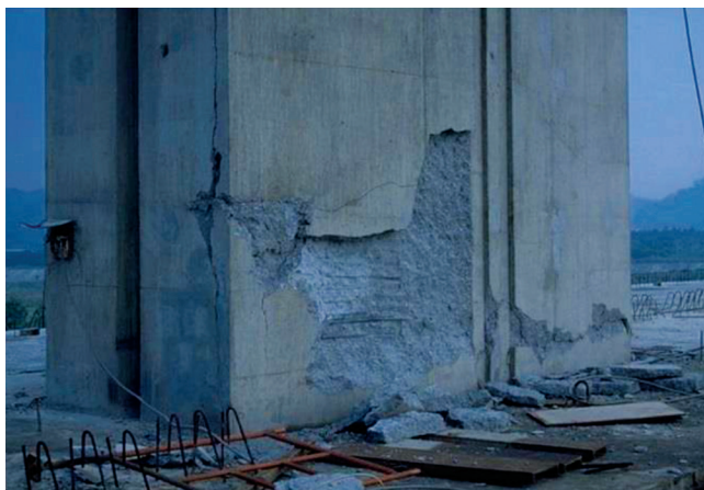
Fig. 4.2.2d—Spalling of concrete at main pylon of the Jyi-Lu Bridge, Chi-Chi Earthquake 1999. (Courtesy of NISEE, University of California, Berkeley, CA [Moehle 1999a].)
