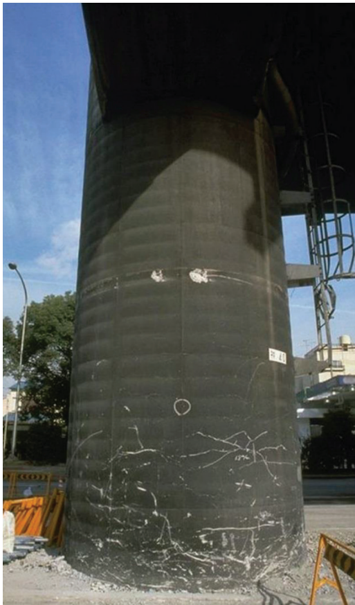
Fig. 4.2.2a—Cracking and spalling, circular column, Pier 40 of the Hanshin Expressway, 1995 Kobe Earthquake. (Courtesy of NISEE, University of California, Berkeley, CA [Thewalt 1995b].)
