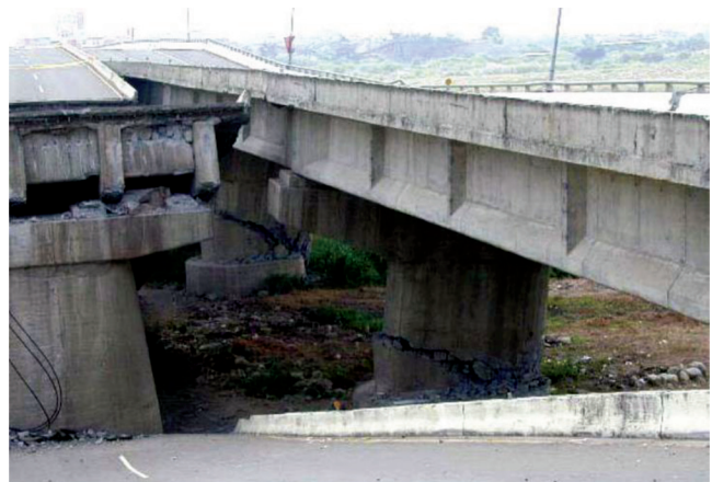
Fig. 4.2.4j—Column shear failure and loss of seat support, Wu-Hsi Bridge, 1999 Chi-Chi Earthquake. (Courtesy of NISEE, University of California, Berkeley, CA [Moehle 1999c].)
