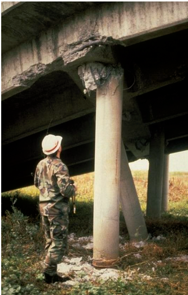
Fig. 4.2.4h—Pile failures, Highway 101 at Struve Slough, 1989 Loma Prieta Earthquake. (Courtesy of NISEE, University of California, Berkeley, CA [Boulanger 1989b].)
