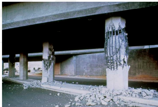
Fig. 4.2.4b—Shear failure of several columns, possibly associated with deck rotation, Foothills Freeway overpass, 1971 San Fernando Earthquake. (Courtesy of NOAA/NGDC, U.S. Geological Survey [Leyendecker 1971a].)
