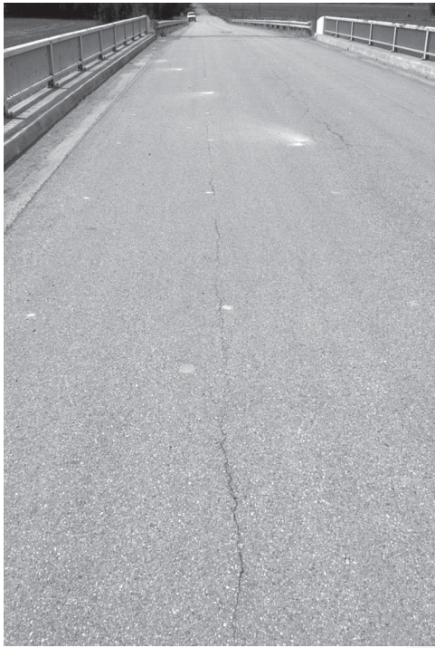
Fig. 4.1f—Deteriorated asphalt wearing surface.
