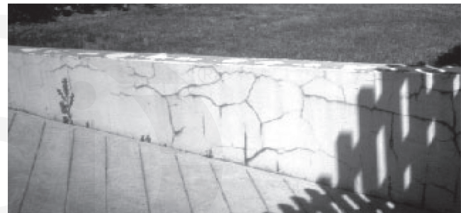
Fig. 4.1d—Map cracking in parapet.
