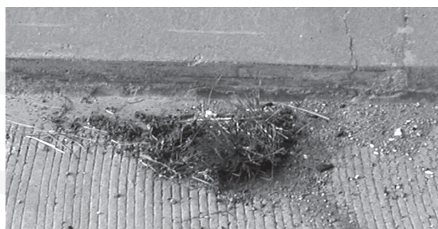
Fig. 5.2.2b—Plugged deck drain.
