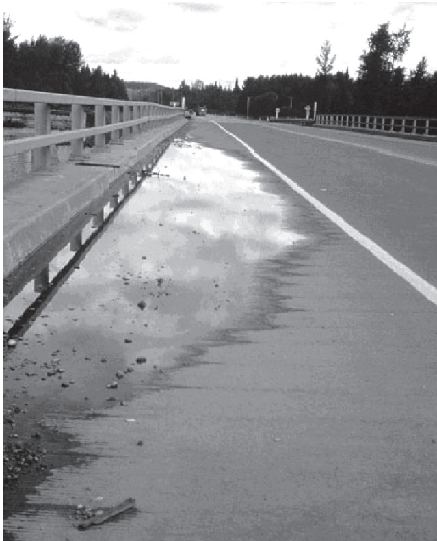
Fig. 4.1a—Water ponding from improper deck drainage.
