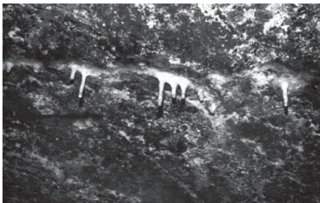
Fig. 4.3.4—Efflorescence from freezing-and-thawing deterioration.
