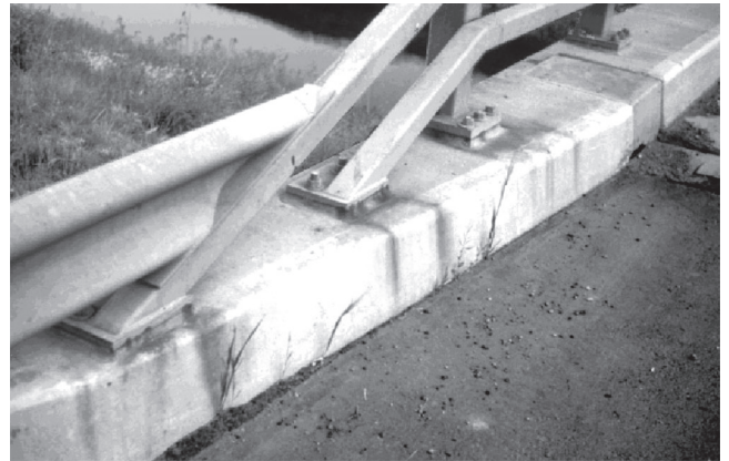
Fig. 4.1h—Rust staining of curb.
