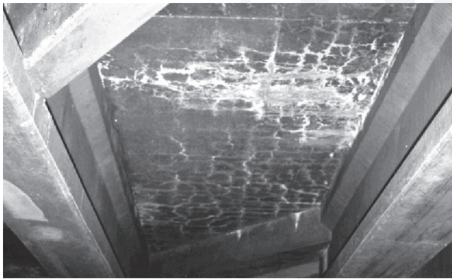
Fig. 4.1b—Map cracking on underside of deck.
