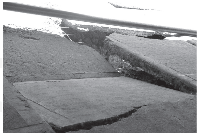
Fig. 4.1i—Erosion and settlement of slopewall.
