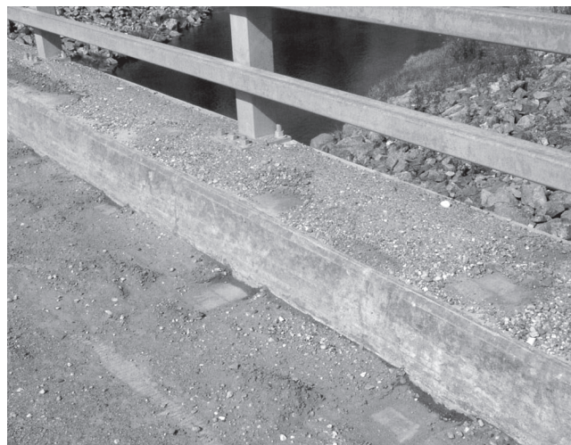
Fig. 5.2.2a—Debris accumulation on curb.
