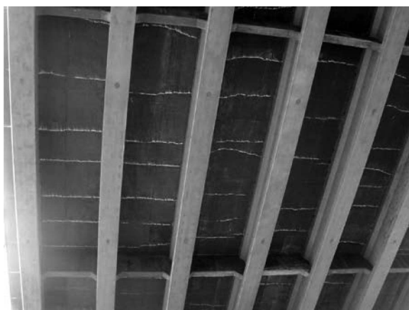
Fig. 3.4.3—Transverse cracking (from below).
