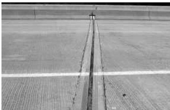
Fig. 3.7.4—Typical strip seal joint system in service.
