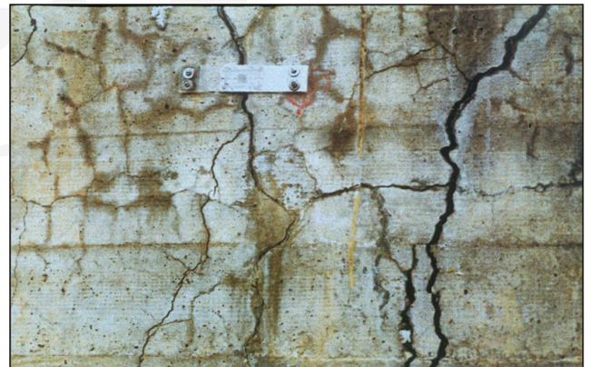
Fig. 2—Monitoring changes in crack width.
