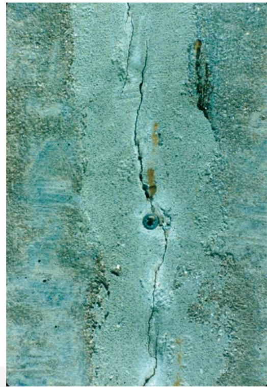
Fig. 2—Example of an active crack improperly repaired.
