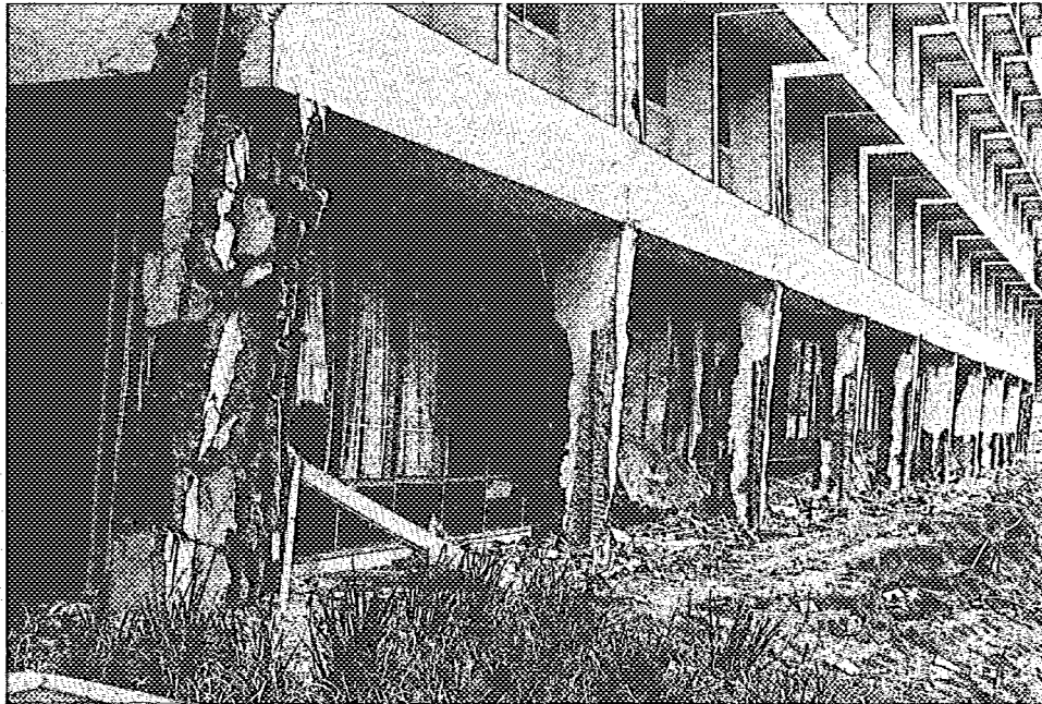
Fig. 1.3.3(a)—Damage caused by San Fernando earthquake (Los Angeles, 1971)
