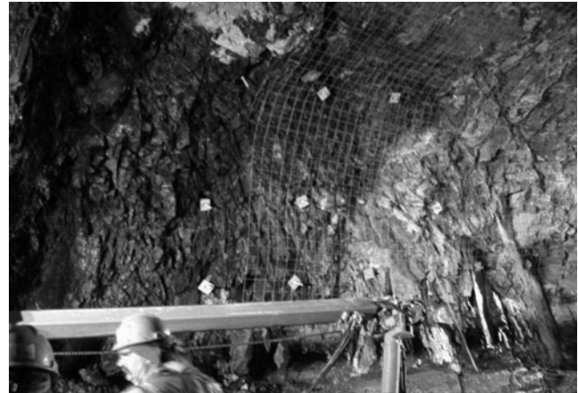
Fig. 5.4—Wire mesh in tunnel with considerable overbreak.
