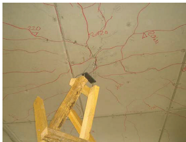
Fig. 5.2—Distributed cracking under full-scale elevated slab subjected to concentrated load (location: Tallinn, Estonia, 2007) (photo by courtesy of X. Destrée).
