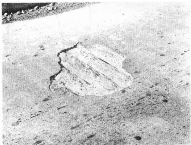
Fig. 3 – A typical spalled area (courtesy National Research Council, Transportation Research Board).
