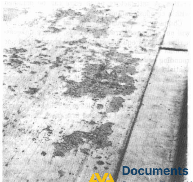
Fig. 5 — Scaled concrete (courtesy Portland Cement Association).
