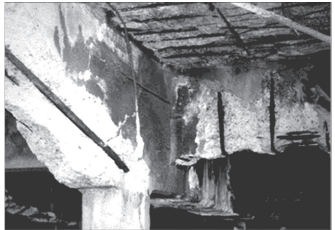
Fig. 3.5.1—Spalled and cracked concrete attributed to corrosion of the steel reinforcement (image courtesy of Collins Engineers, Inc.).
