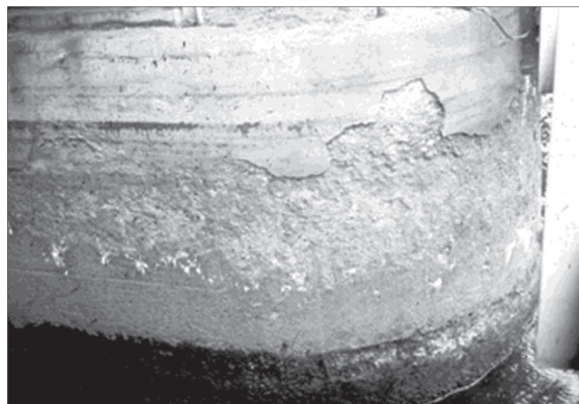
Fig. 3.7—Concrete deterioration on a bridge pier attributed to cycles of freezing and thawing (image courtesy of Collins Engineers, Inc.).
