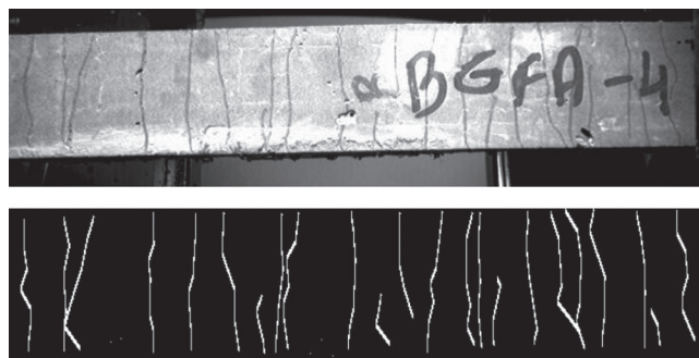
Fig. 3.2.1b—Distributed cracking in AR-glass-FRCM (width = 1 in. [25 mm]).
