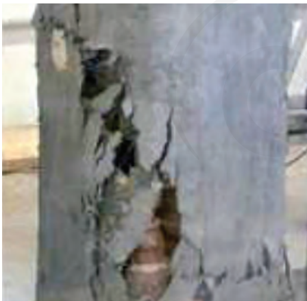
Fig. 3.4.3a—Failure by tensile rupture of the basalt FRCM and crushing of the confined column (Fossetti et al. 2016).
