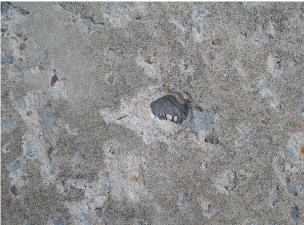
Fig. 2.7—A popout occurs when internal pressure causes a small part of the concrete surface to break away, usually leaving a cone-shaped hole. Popouts range in size from 1/4 in. (6 mm) or less in diameter to 2 in. (50 mm) or more, depending on aggregate size (photo courtesy of Frances Griffith)
