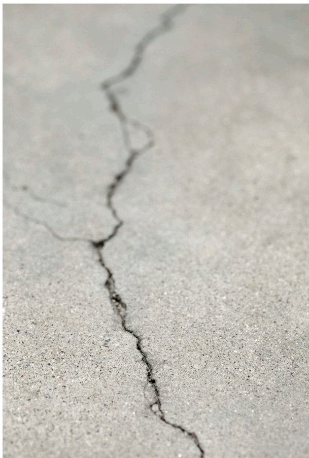
Fig. 1.10—Concrete cracking can be unsightly and depending on the location can reduce the service life of the structure
