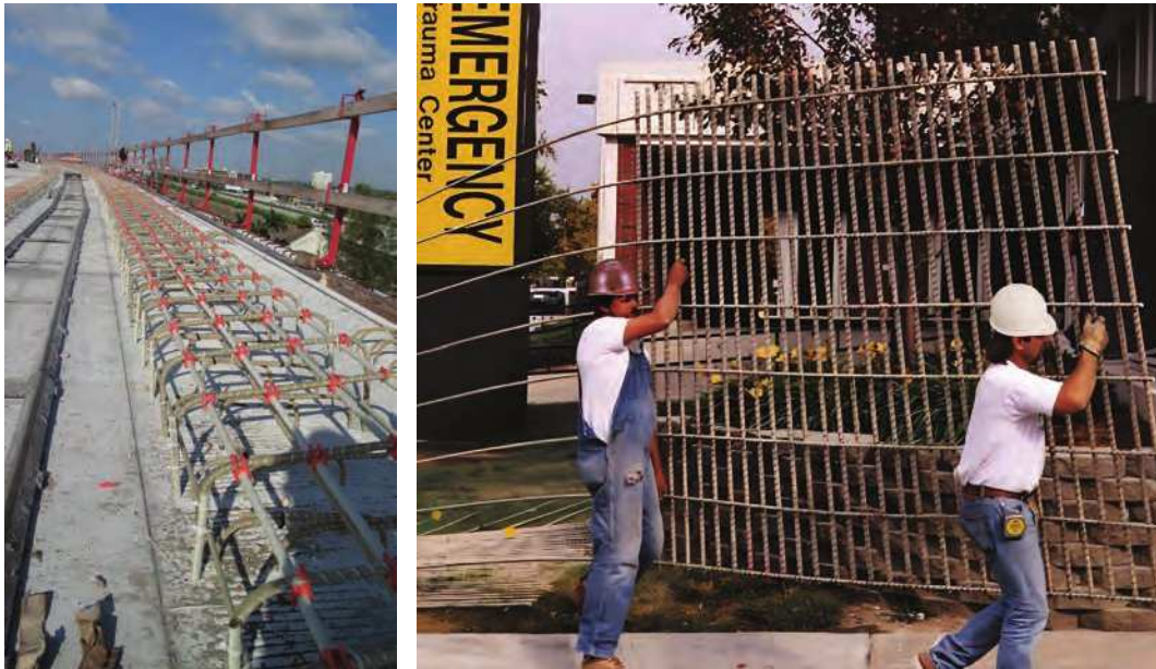
Fig. 1.1a—GFRP reinforcement used around MRI units in hospitals and in maglev train applications. The photo on the left is of the AirportLink maglev railway that connects to the Miami Intermodal Center (MIC), built in 2011. The photo on the right is a cage of reinforcement being transported to a concrete placement in a room that will eventually house an MRI unit (photos courtesy of Doug Gremel).
