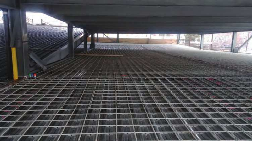
Fig. 3.1.1a—This parking garage uses GFRP reinforcement as the top mat of reinforcement to minimize corrosion issues. Vehicles carrying deicing salts into parking garages can create corrosion issues on the top of parking decks, leading to shortened lifespans of these structures (photo courtesy of Owens Corning Infrastructure Solutions).
