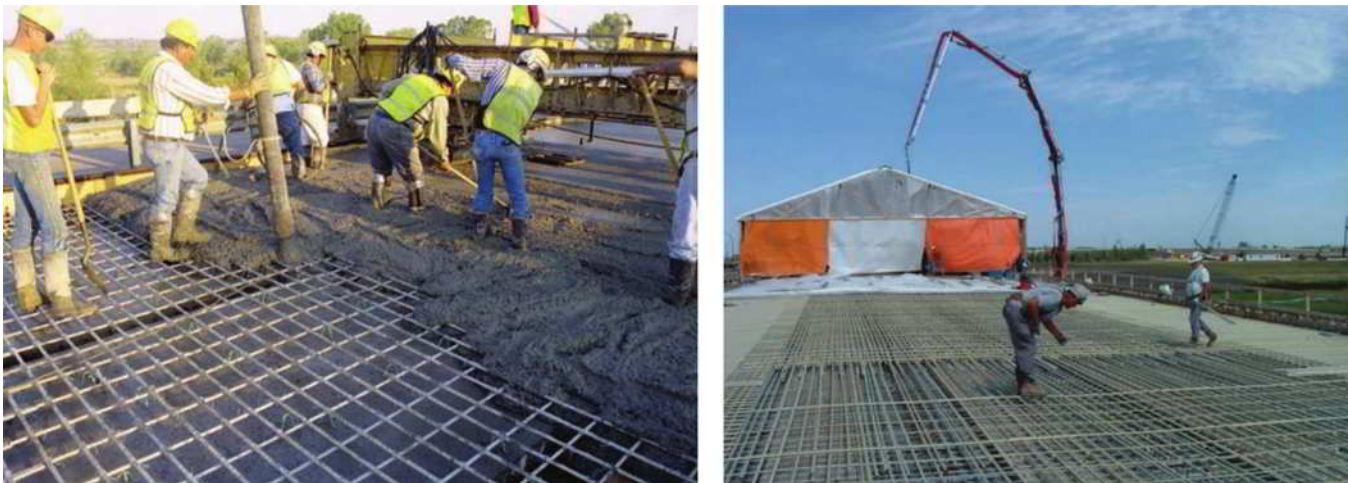
Fig. 5b—Bridge decks reinforced with GFRP bars as a way of mitigating corrosion issues when exposed to deicing salts. The photo on the left is of the Sierrita de la Cruz Creek Bridge in Amarillo, TX, which was constructed in 2000. The photo on the right is of the Floodway Bridge over the Red River in Winnipeg, MB, Canada, which consumed over 310,000 lb (140,000 kg) of GFRP reinforcing bars and was constructed in 2006.
