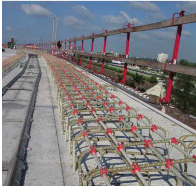
Fig. 3.5—GFRP reinforcement of a structure built to support a magnetic levitating (maglev) train (photo courtesy of Owens Corning Infrastructure Solutions).
