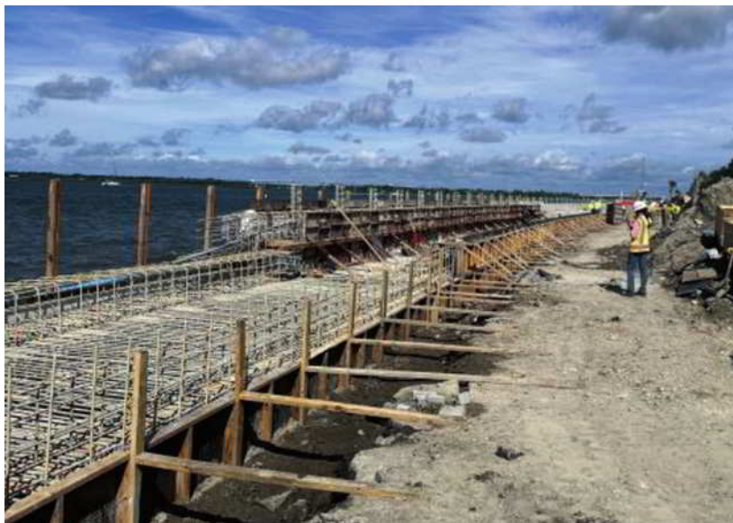
Fig. 3.2—A seawall reinforced with GFRP bars (photo courtesy of Owens Corning Infrastructure Solutions).
