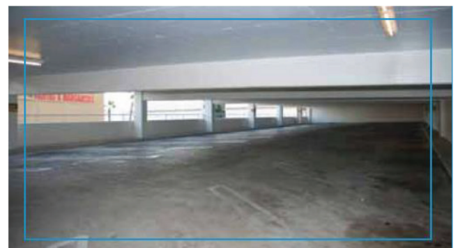
Fig. 5.3a—Parking Structure #2 (Level 4 interior) (Bondy 2011).
