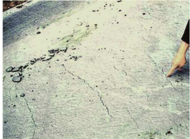
Fig. 4.1.2.7—Plastic shrinkage cracking.
