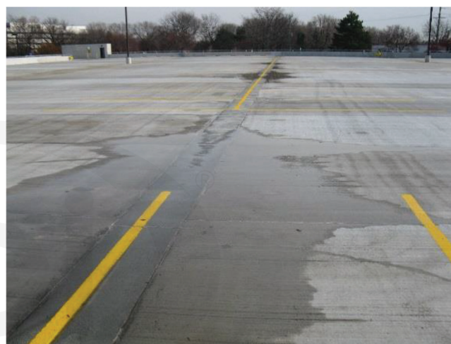
Fig. 2.1.8—Ponded water can contribute to leakage problems and lead to accelerated deterioration.
