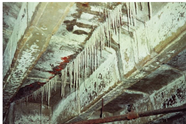
Fig. 2.1.7—Leaking and leaching can result in extreme deterioration conditions if cracks are not sealed.
