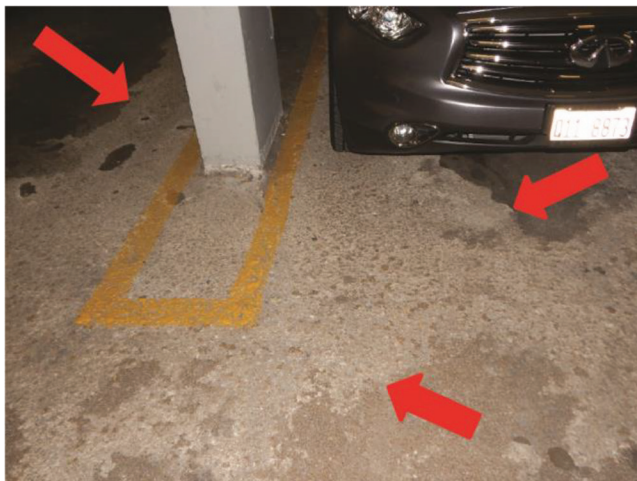
Fig. 2.1.1—Area of scaling on concrete surface.
