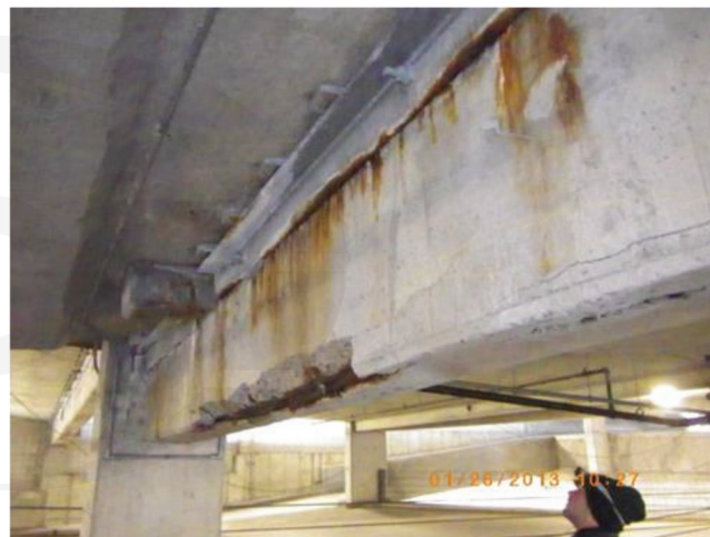
Fig. 2.2.2a—Delamination and spalling on beam beneath leaking expansion joint.
