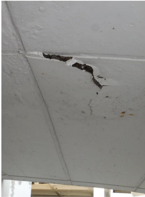
Fig. 2.1.3—Loose delaminated concrete on slab underside.
