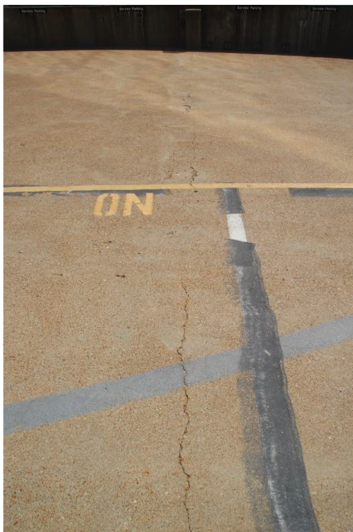
Fig. 2.1.5—Cracks in concrete allow accelerated absorption of water and chlorides.
