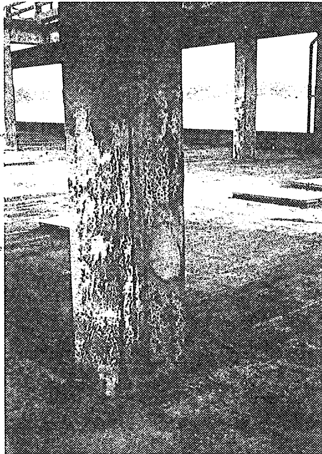
Fig. 1--Photographs showing steel corrosion in structural concrete elements (Hood Canal)
