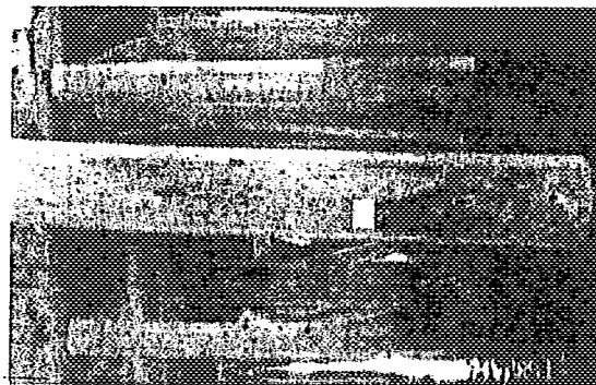
Distressed pile before repair
