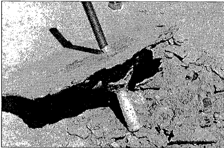
Fig. 8--Bond failure: the bond between the chemical resin or epoxy and the concrete fails, allowing the anchor to pull out. This type of failure is common for chemical anchors embedded between 6.0D and 9.0D, and is usually accompanied by a shallow concrete cone with a depth up to one-half of the stud embedment
