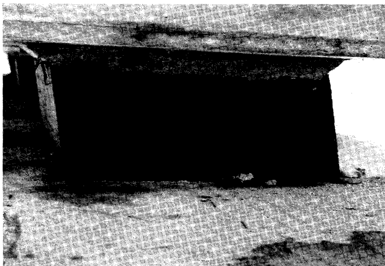
Fig. 26—Creep shrink effect on elastomeric bearing requires jacking and repositioning
