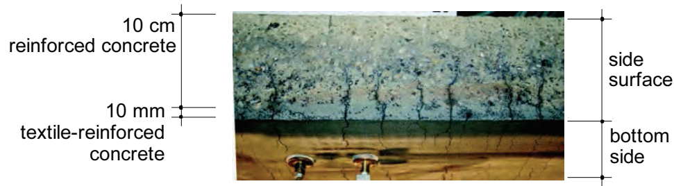
Figure 2 - Crack pattern of flexural TRC-strengthened RC-slab
