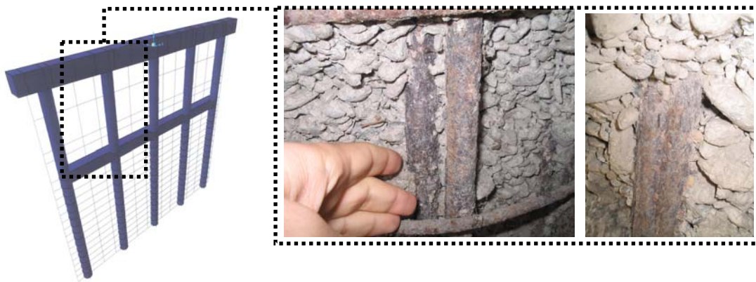
Fig. 5 —Carbonation phenomena, absence of binder and higher maximum diameter of the rubble
