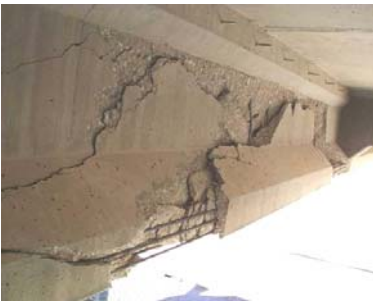
a) The impact damaged beam.
