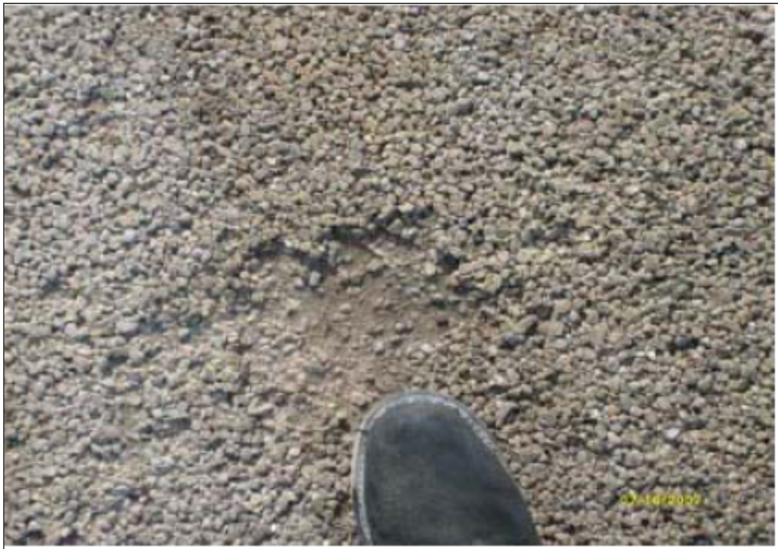
Figure 1 – example of raveling
