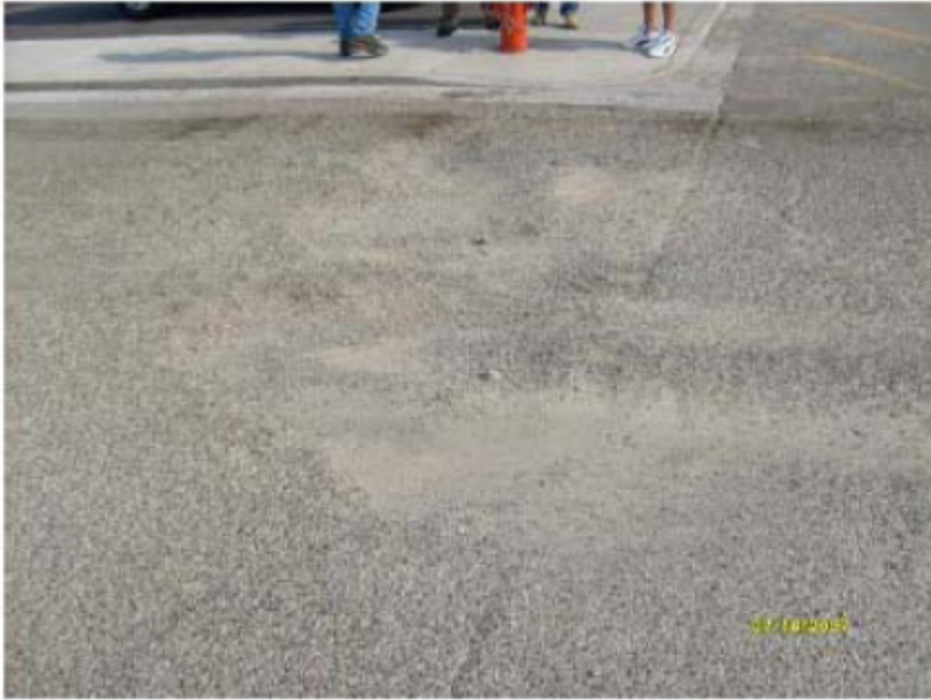
Figure 12 – Heavy Vehicle Damage
