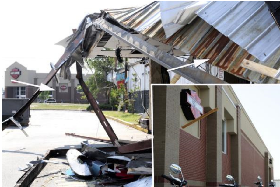
Fig. 4—During a tornado in Georgia, this awning was ripped apart and board was impaled into an adjacent concrete wall (inset) (photo courtesy of Mike Moore, FEMA)
