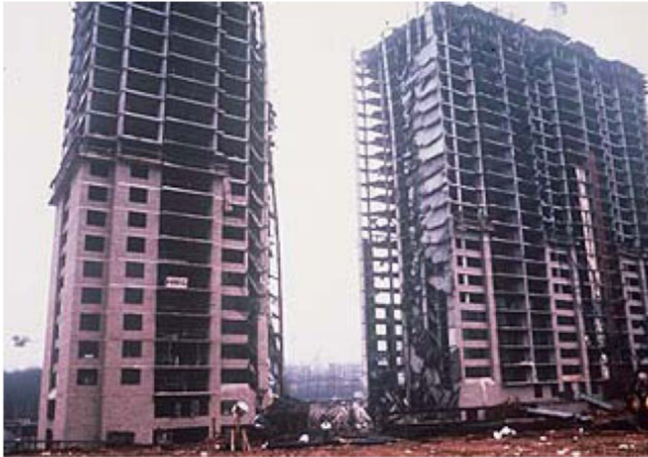
Figure 3 – Skyline Plaza/ Bailey's Crossroads Collapse (photo courtesy Nick Carino of NIST)
