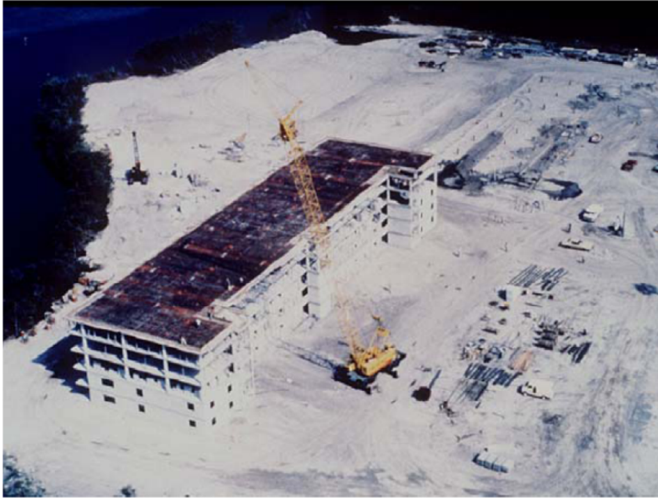
Figure 5 – Harbour Cay Condominium before Collapse (photo courtesy Nick Carino of NIST)
