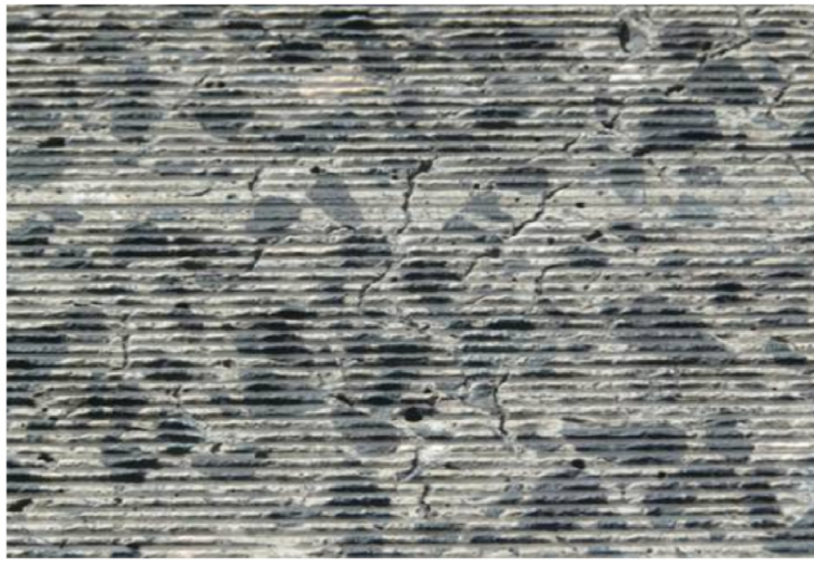
Figure 5 – Plastic shrinkage cracks
