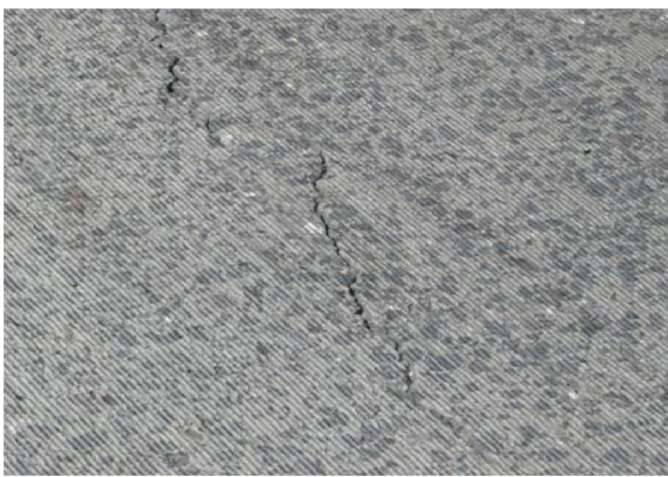
Figure 6 – Full depth cracks
