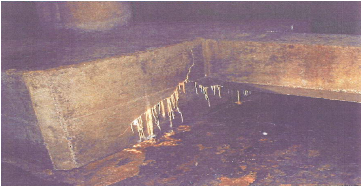
Figure 3-- Cracks in the foundation system following the earthquake
