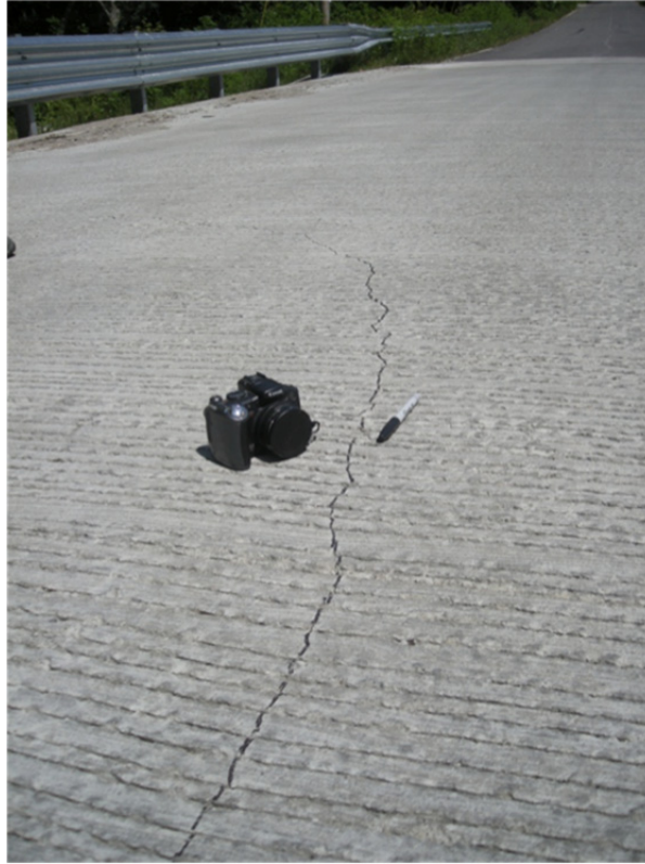
Figure 4—Cracking in conventional concrete bridge deck after 3 months of service 30
