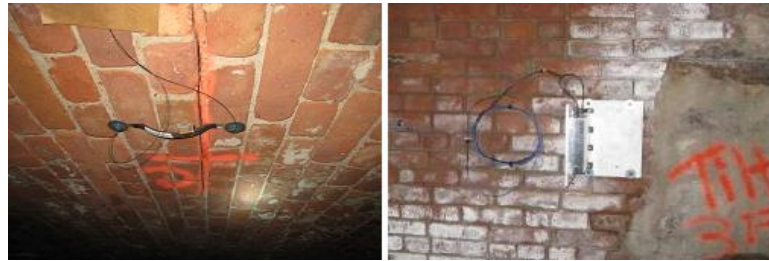
Figure 6 – Typical crack sensor at the crown crack and tiltmeter at the center wall
