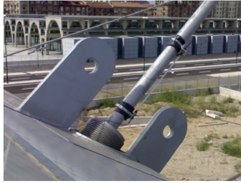
Figure 11 – Typical field installation of FBG cable sensor (LingottoLingotto Bridge).
