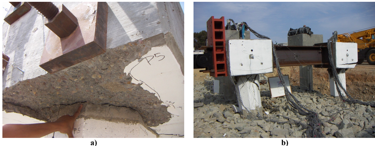
Figure 4 -- Extent of Damage for System Test 1. a) Cap Concrete Spalling. b) Damage Spread to Piles.
