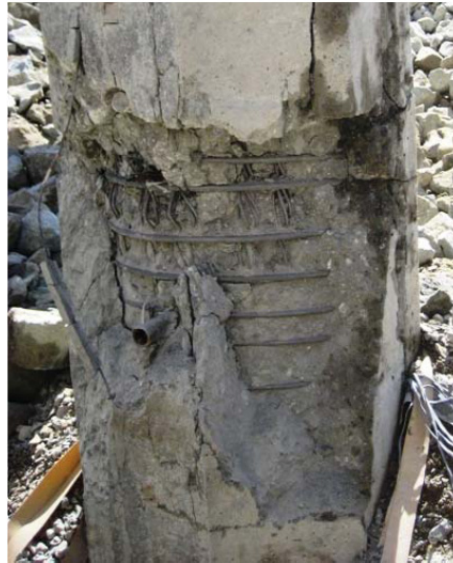
Figure 5 -- Extent of Damage After Excavation in the Level Ground Pile of System Test 1.
