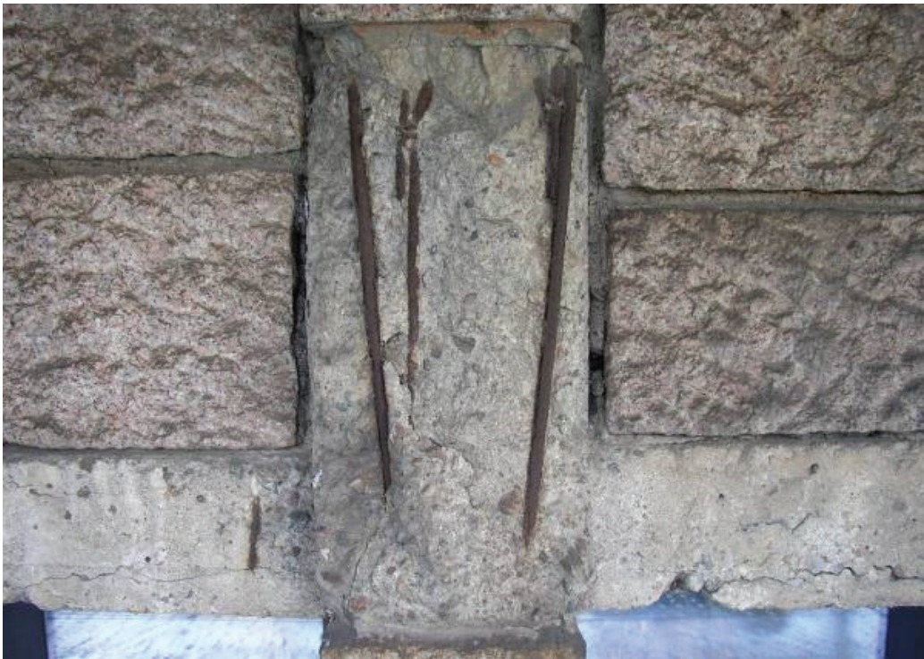
Figure 2–Thickness of concrete cover is less than 10 mm (0,39 in)
