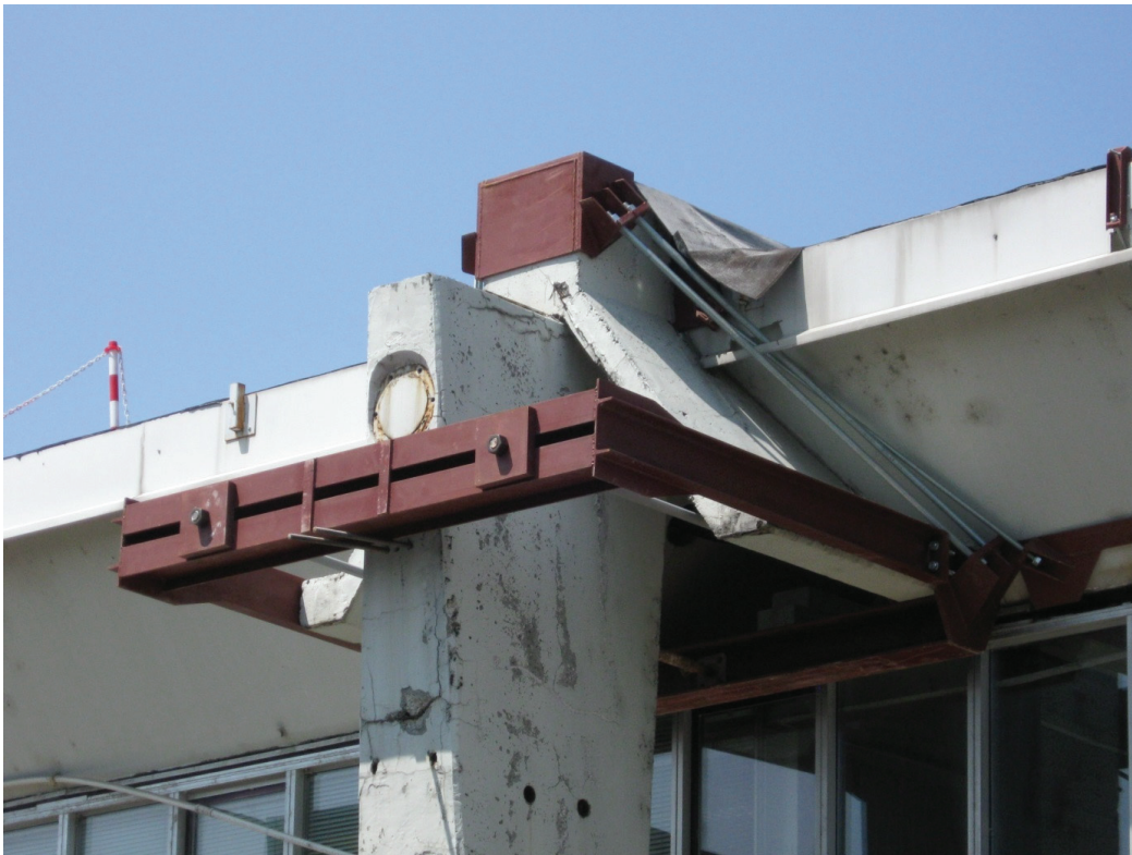
Figure 7 – Connection between pillar and Y-shape beam. Detail of the decay of concrete structures CONCLUSIONS
