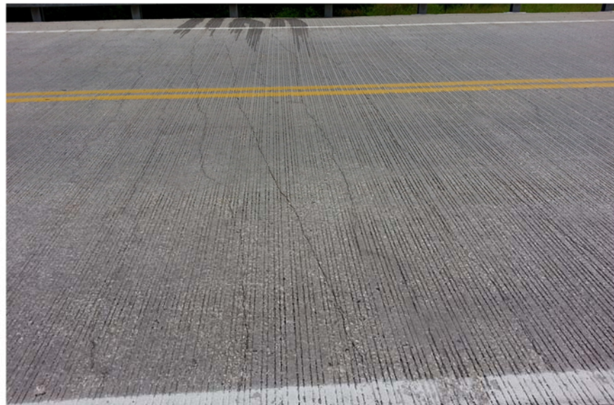
Figure 2 – Extensive wide cracks over the piers of one of the surveyed bridges
