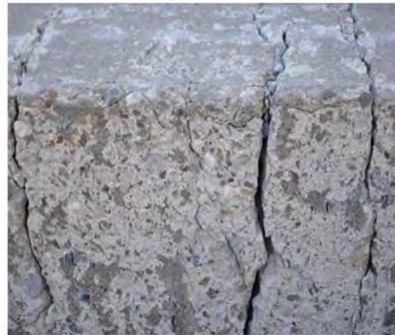
The upside down beam after removing the FRP sheet
