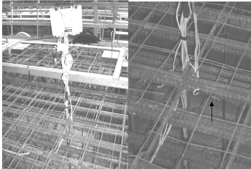
Figure 8 Maturity sensors and centralized monitoring junction box.
