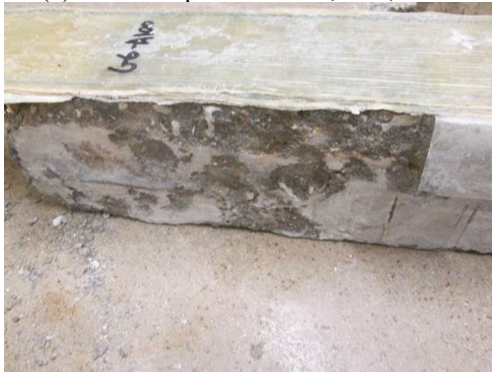
(c) Scaling induced loss of bonded area
