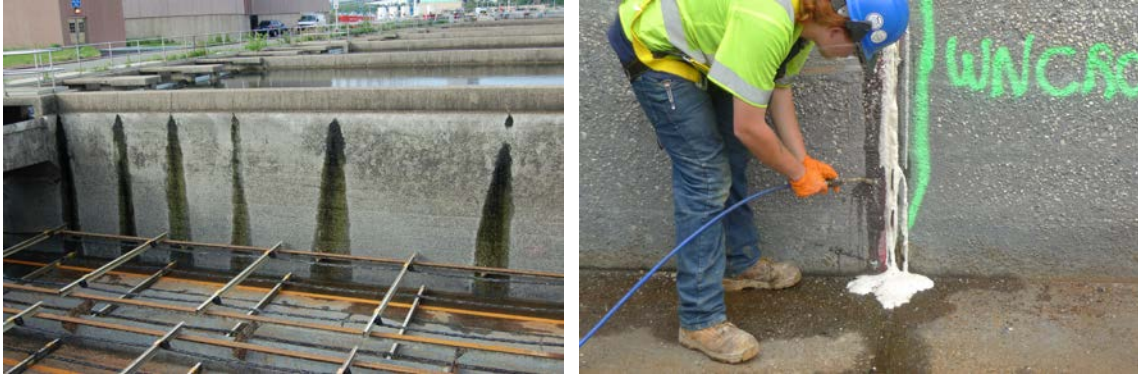
Figure 5 - Cracked tank wall. Water leaks from adjacent tank. Chemical grout injection.
