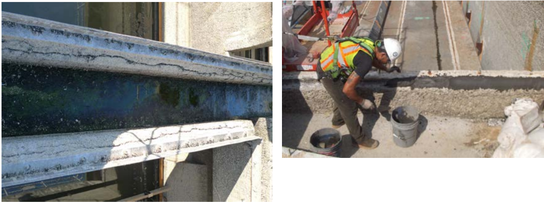
Figure 6 – Cracked troughs and repairs.
