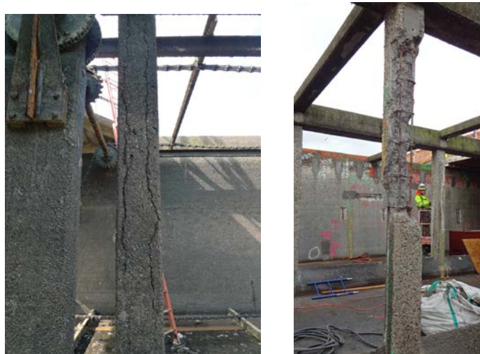
Figure 1 – Cracked and spalled concrete columns and repairs.
