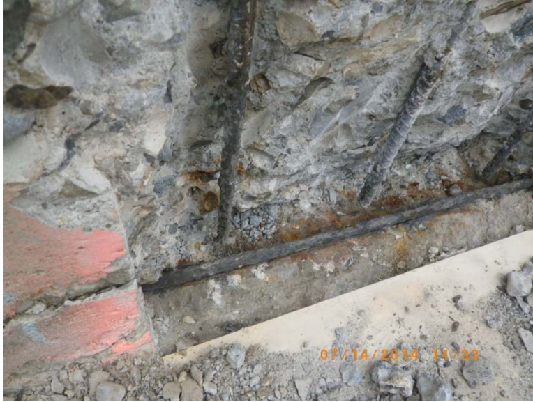
Figure 2 - Reinforcing steel corrosion damage at the base of wall section.
