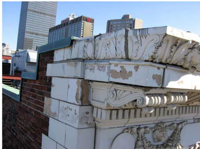
Figure 3 - Projected terra cotta façade elements exhibiting damage consistent with failure of internal supporting steel structure.
