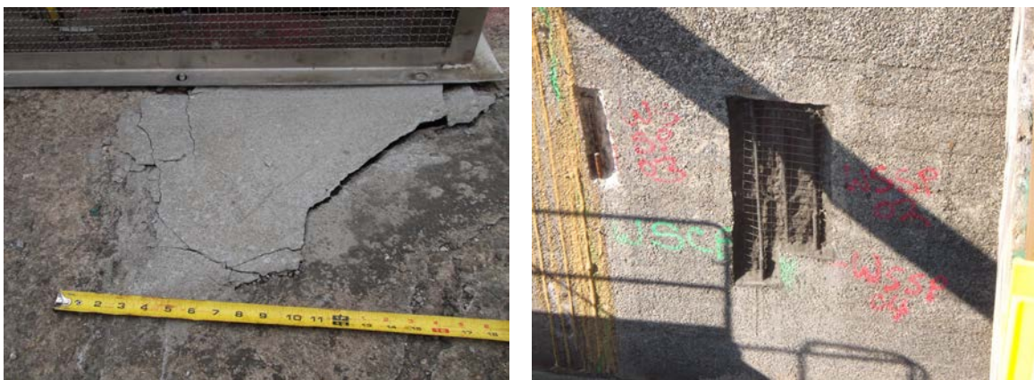
Figure 4 - Spalled concrete and repairs
