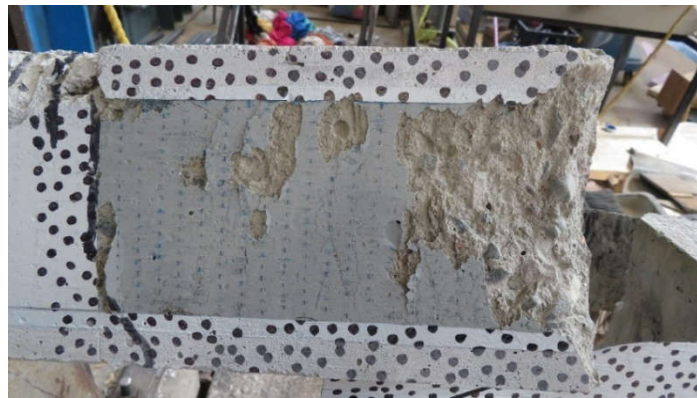
b) Dynamic test with mainly adhesive failing.
