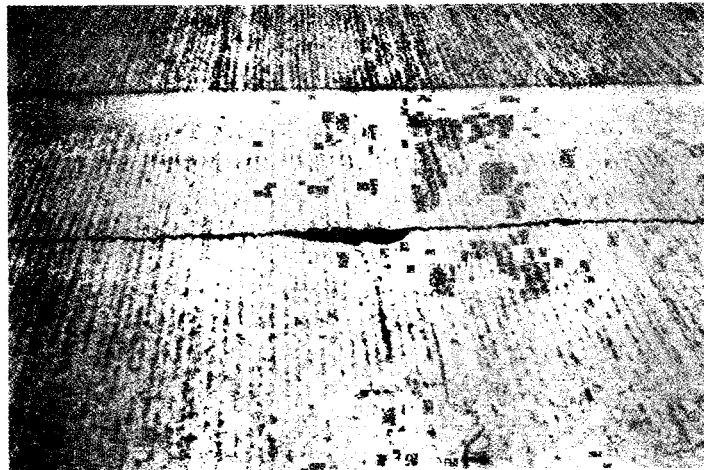
Photo 10—Spalling at intersection of transverse and longitudinal crack (section IV)
